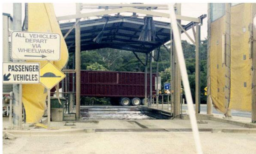
Figure 3.1: Automated wash bay located in a landfill site
