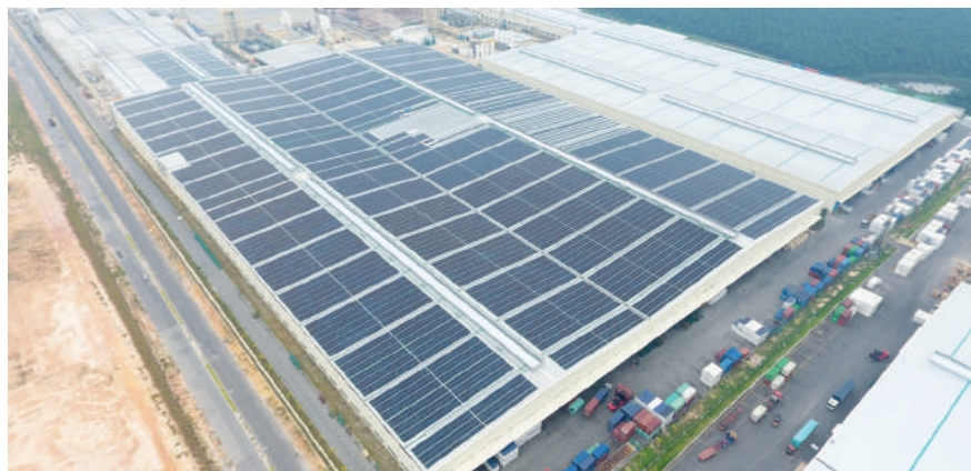
Malaysia’s largest rooftop solar PV project under NEM 2.0 at 31 MWp by Xinyi Solar.
