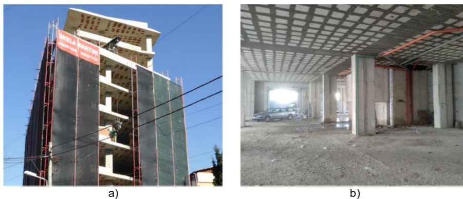
Figure 2. Typical examples of RC frame buildings in Albania: a) a building during construction, b) interior of an existing building
