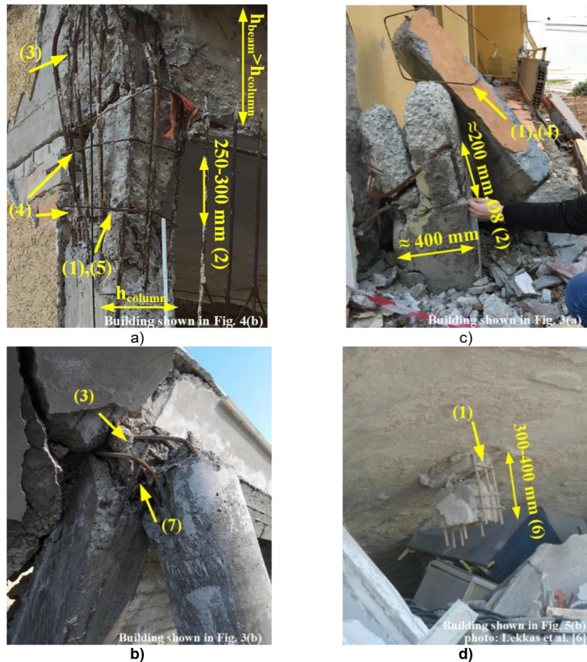
Figure 6. Examples of inadequate detailing of reinforcement in RC columns and beams
