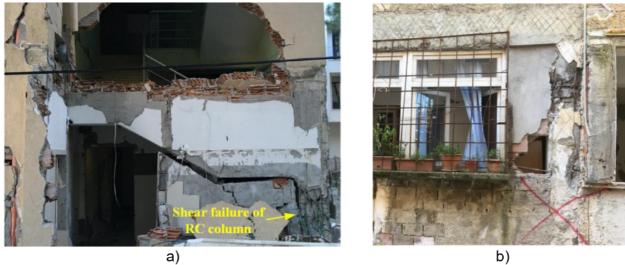
Figure 4. Examples of RC column damage due to “short column” effect in the Albania earthquake caused by: a) intermediate staircase landing, b) partial masonry infill due to openings
