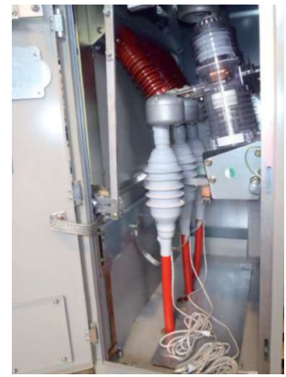
Figure 2.4 – Smart termination installed in a MV/LV substation
