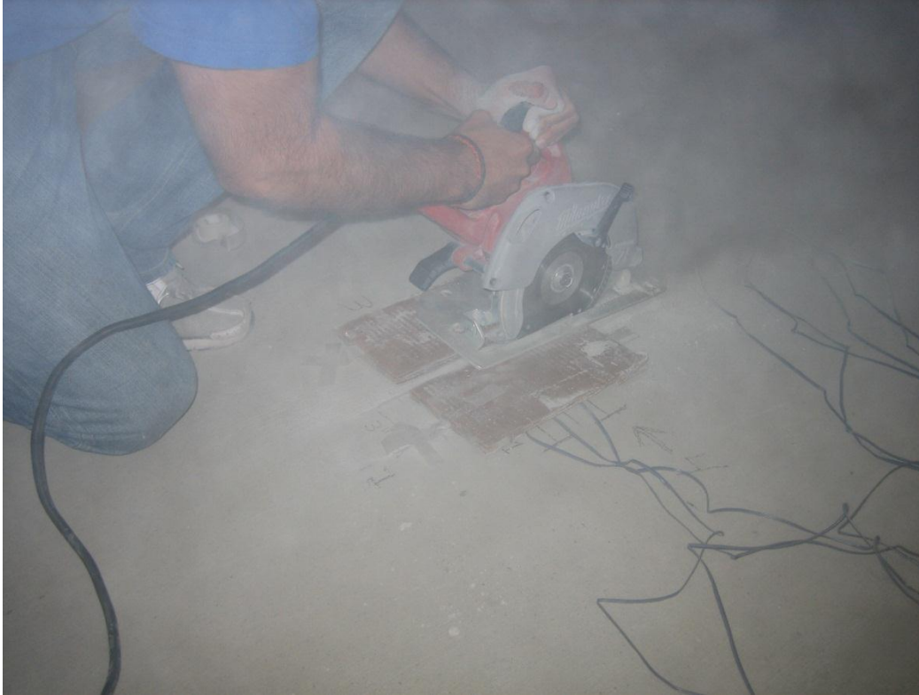
Figure 4.37 Center of saw blade advanced 10 inches forward to the end of the guide line
