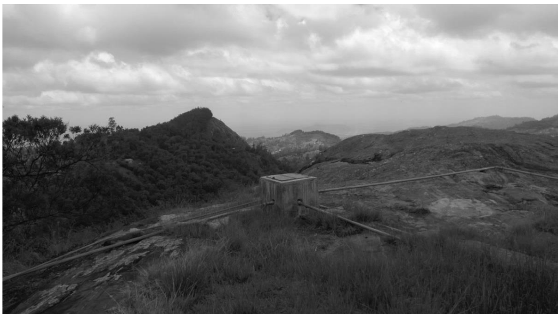
Figure 15. In many cases, the maintenance of the water structures falls on the community members themselves, who might not have the technical knowledge or funds to repair the water infrastructure. These pipes on the top of Kiangungu hill were leaking in February 2013 and thus a village nearby had been without water supply for three weeks (Kivivuori 2013)
