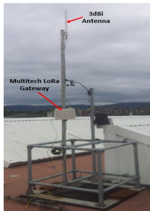
Fig. 2. LoRaWan Gateway installation
