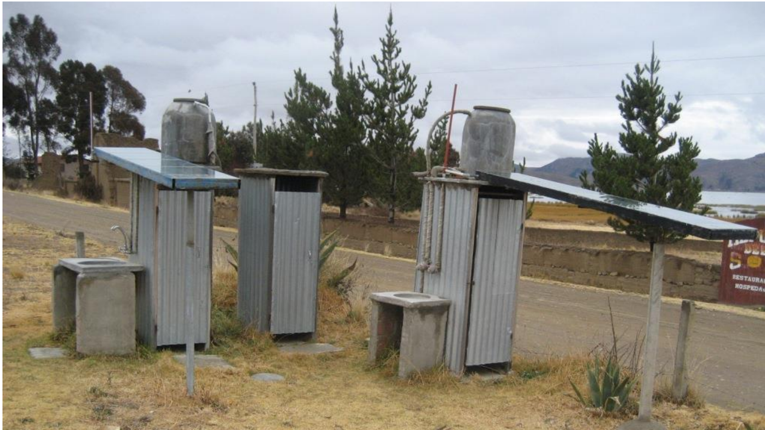
Shower Units at training centre with water pumped through solar water panels
