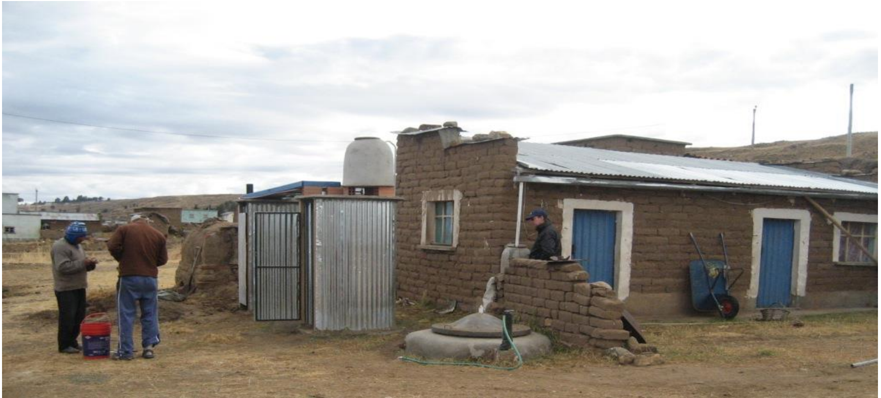
Family rainwater harvesting water supply system
