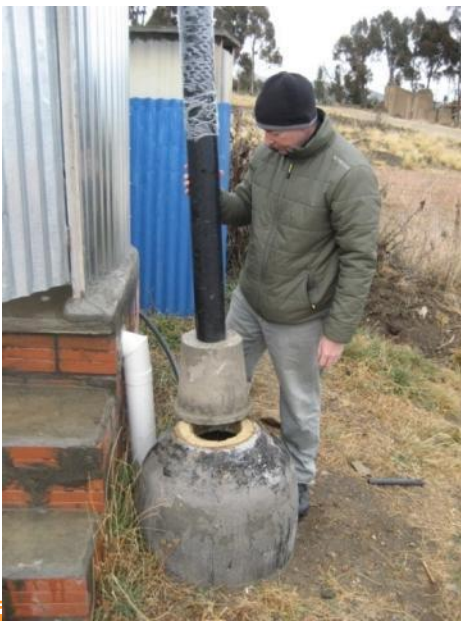
Latrine odour removal system using straw material housed in an air chamber
