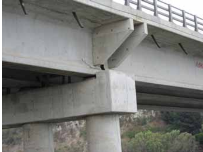
Figure 3.34 Shearing of bridge girder, north abutment of bridge, Puente Mataquito, April 16, 2010 (-35.050712°, -72.162258°)
