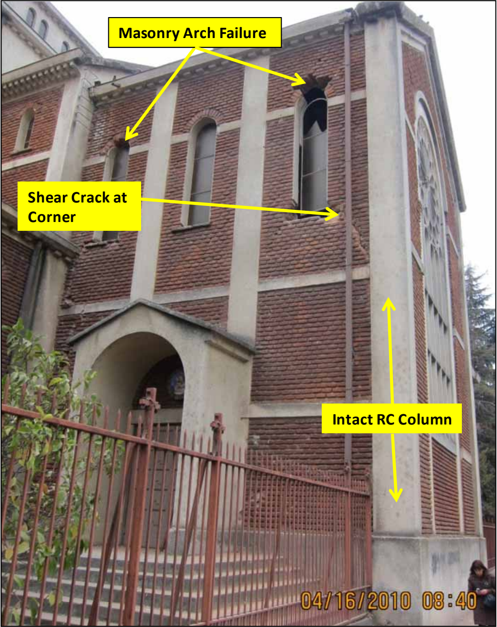
Figure 4.94 Exterior damage to masonry walls
