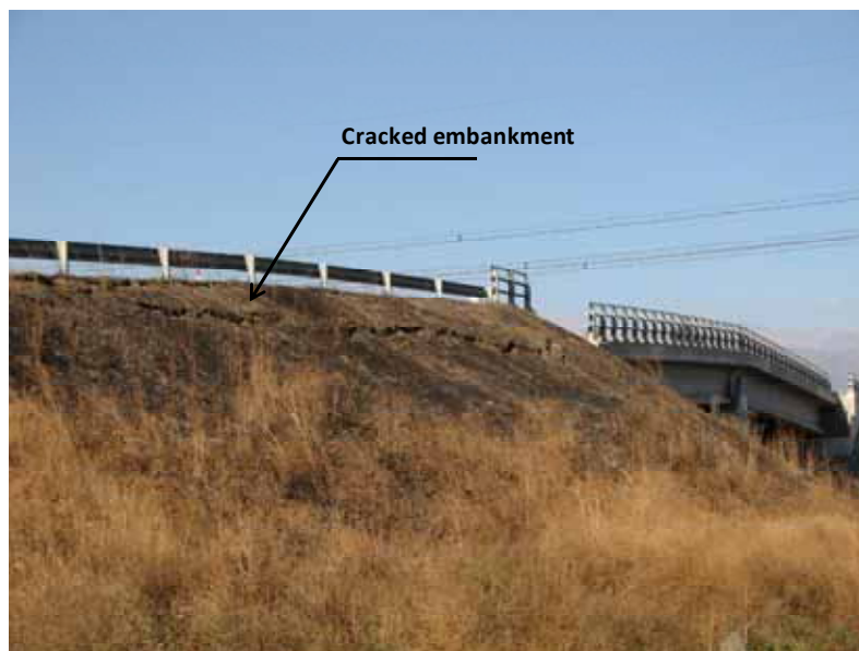
Figure 3.35 Surface cracks at the embankment of Las Mercedes Bridge
