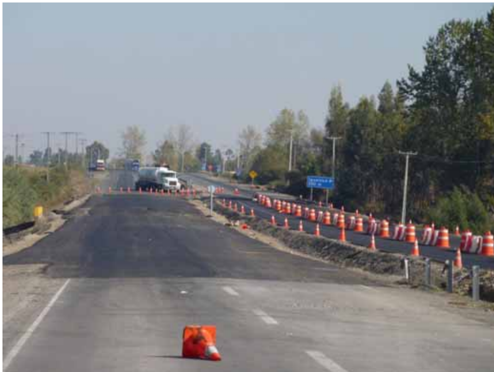
Figure 3.22 Northbound lane looking south, Repaired Roadway Embankment ~5km south of Parral, Route 5 South, April 15, 2010 (-36.185671°, -71.825415°)
