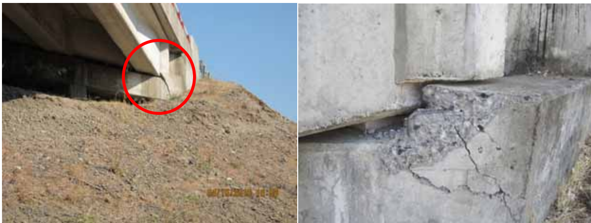
Figure 4.59 Failure of the shear keys
