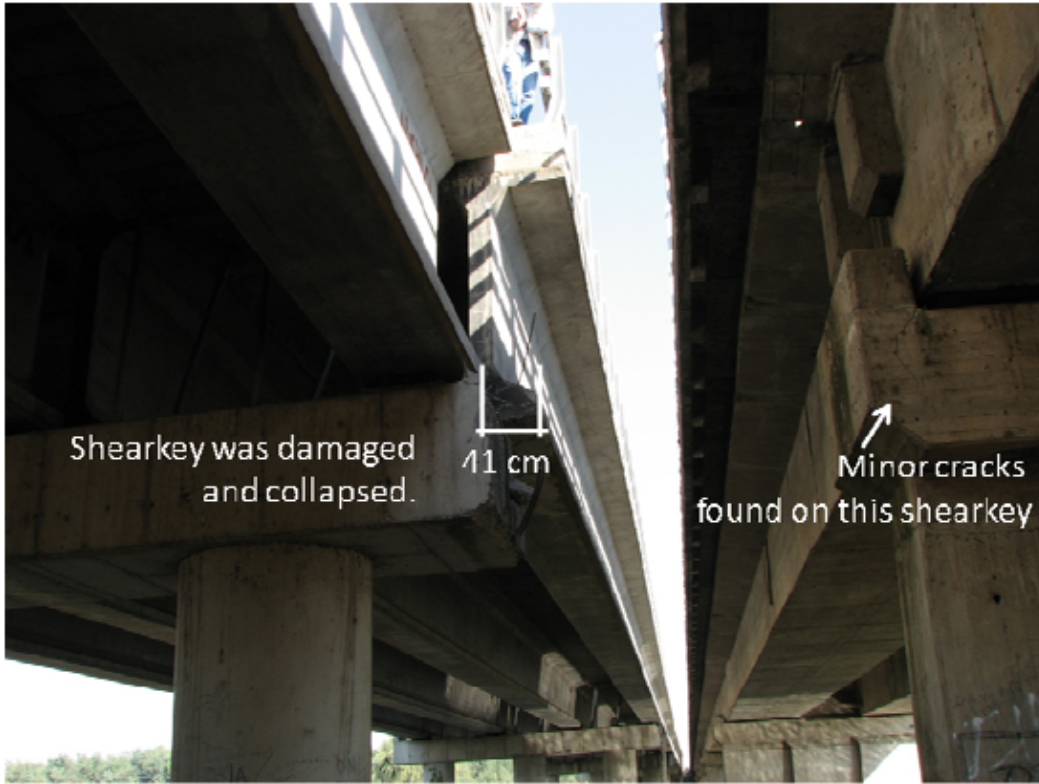
Figure 4.49 Displaced bridge superstructure and damage on shear keys
