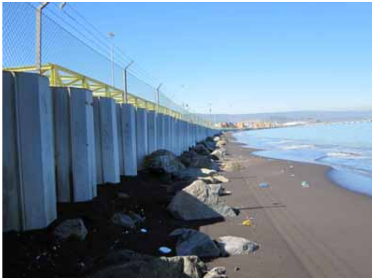
Figure 3.13 Seaside view of the sheet pile wall that experienced lateral spreading, Port of Coronel, April 14, 2010 (-37.028874°, -73.149768°)
