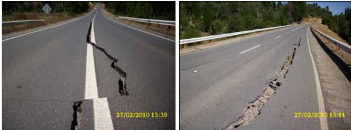
Figure 5.5 Pavement damage due to embankment slope stability and lateral spreading
