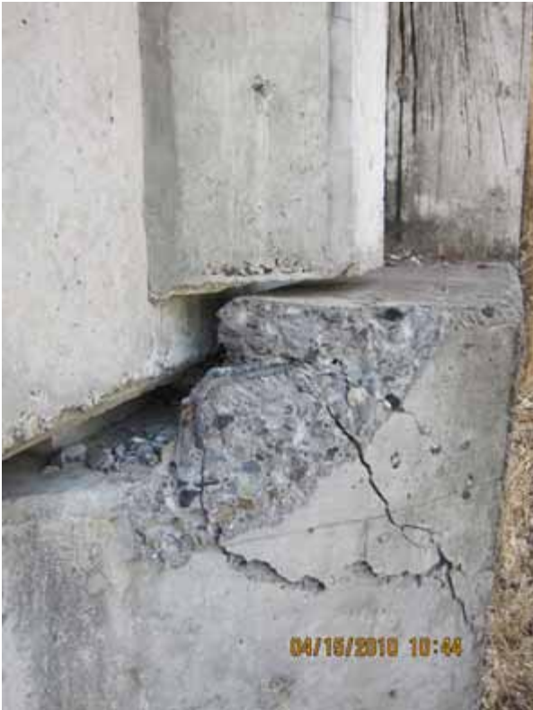
Figure 4.53 Damaged shear key at abutment
