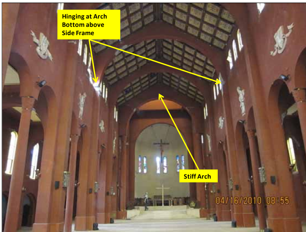
Figure 4.100 Interior damage to high columns at junction with side isles
