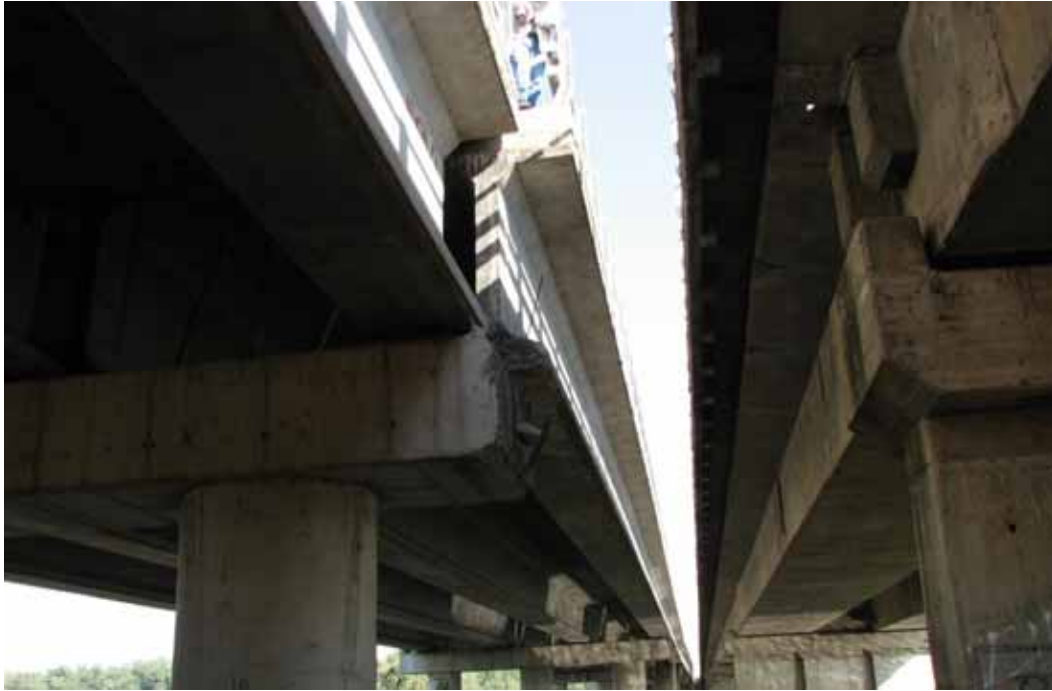
Figure 4.51 Bridge girder close to unseating
