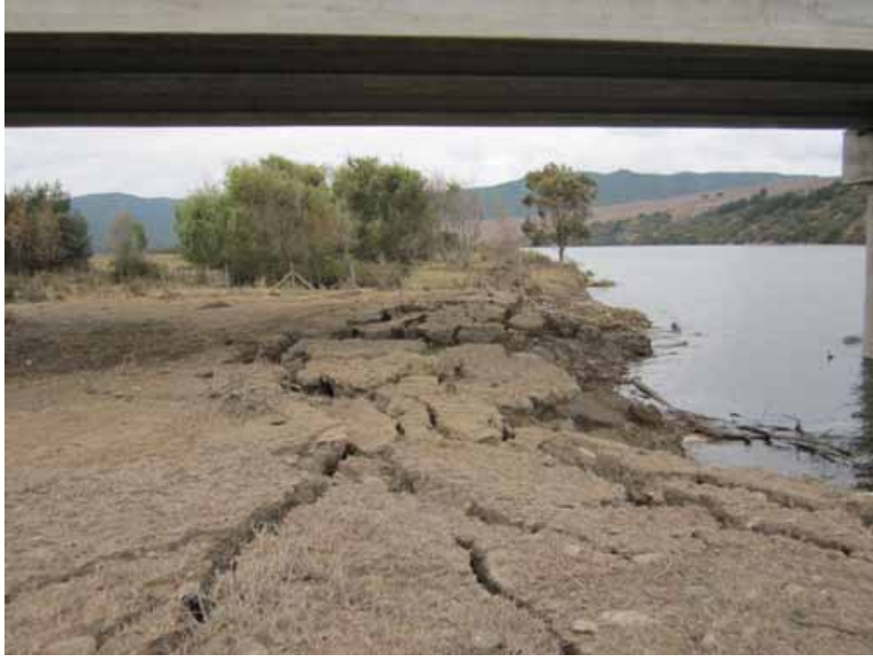
Figure 3.32 Lateral Spreading towards the river, north abutment of the bridge, Puente Mataquito, April 16, 2010 (-35.050712°, -72.162258°)
