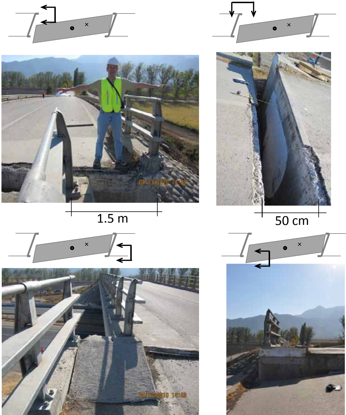
Figure 4.45 Translation of bridge superstructure
