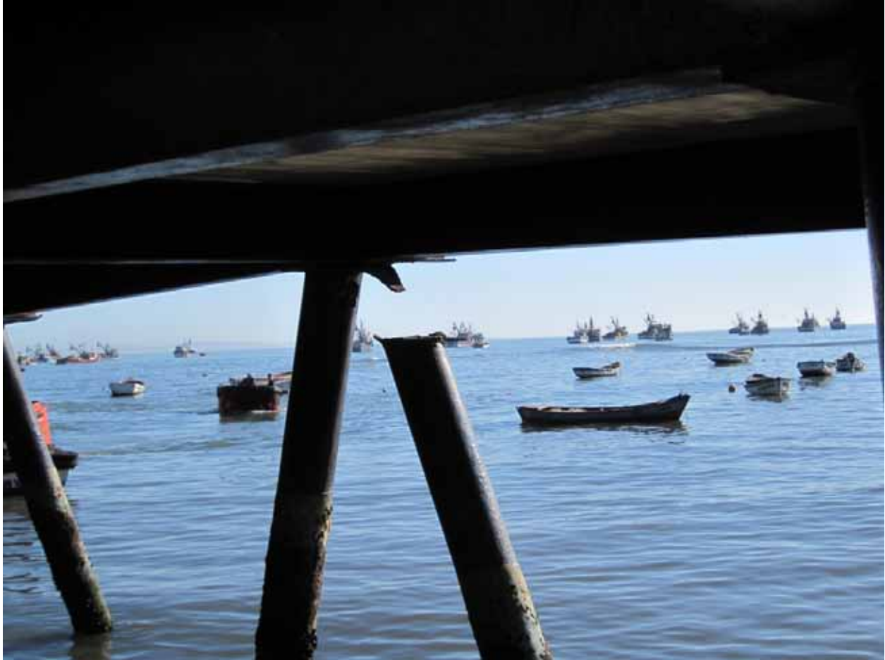
Figure 3.16 Typical broken pile connections, Port Lota, April 14, 2010 (-37.097295°,-73.159331°)
