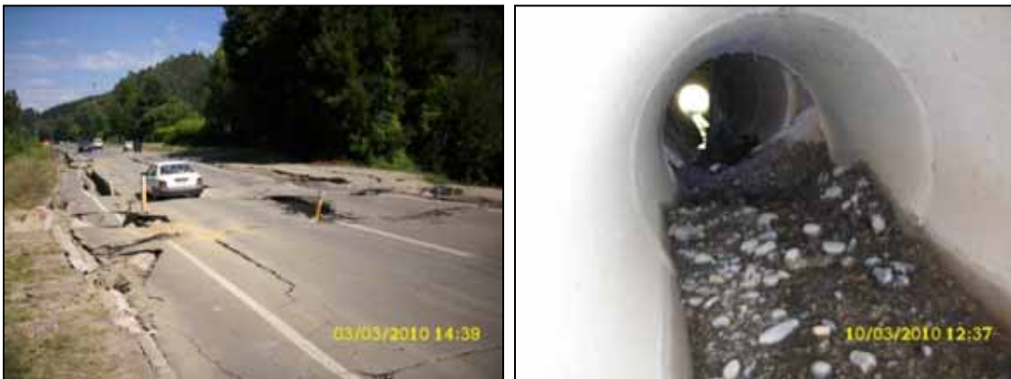
Figure 5.4 Left: under-drain fill settlement at the roadway surface; Right: collapsed drainage pipe
