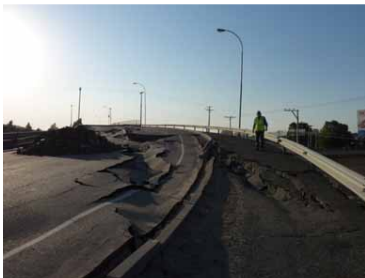
Figure 3.24 Damage to overpass embankment, Route 5 South overpass embankment, to Retiro at Tucapel Mill, April 15, 2010 (-36.051209°,-71.768005°)
