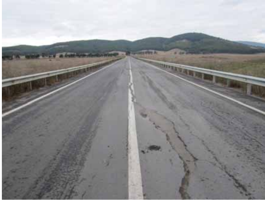
Figure 3.30 Cracking and transverse movement (60 cm on each side) of embankment due to liquefaction of underlying soil, north abutment of the bridge, Puente Mataquito, April 16, 2010 (-35.050712°,-72.162258°)
