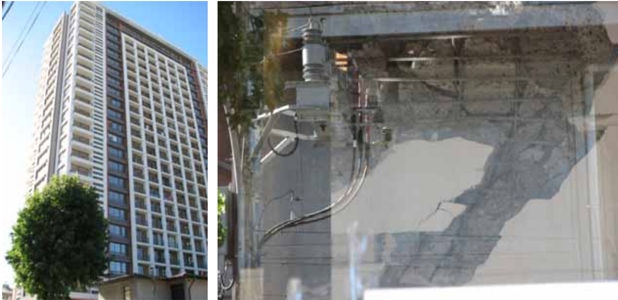
Figure 4.17 Severely damaged condominium high-rise building in Concepción
