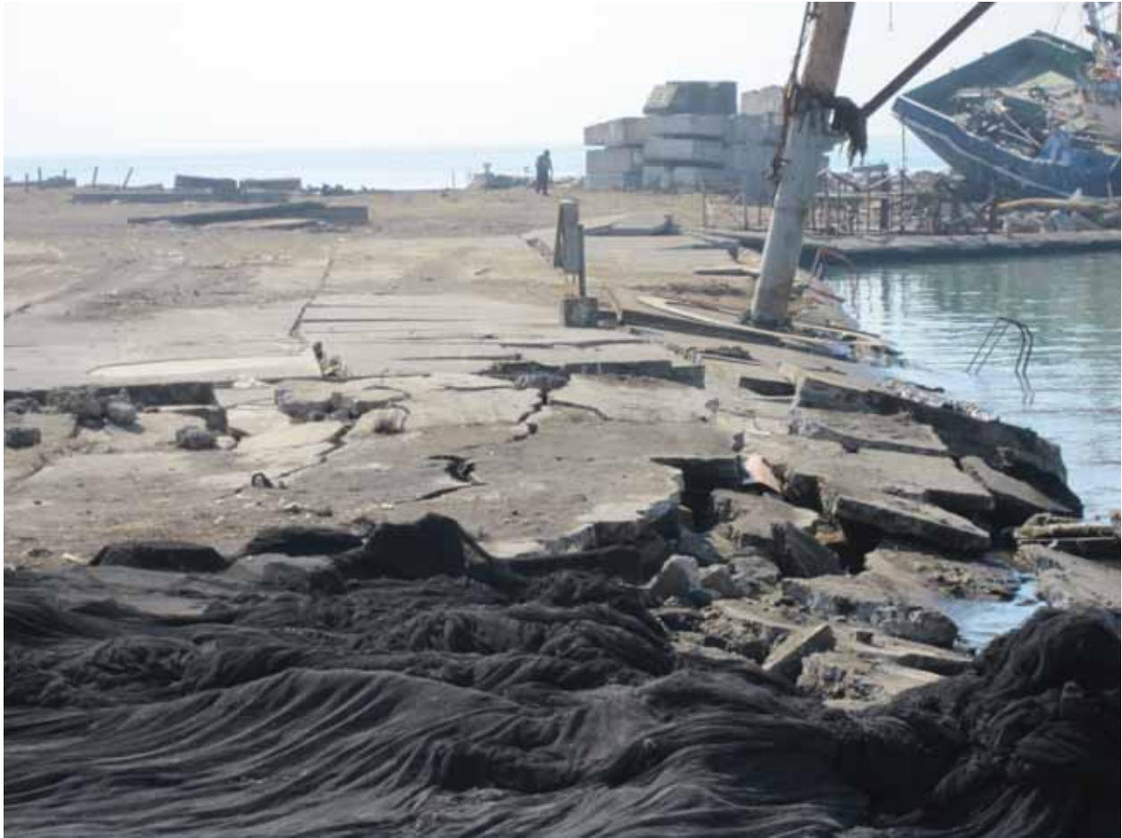
Figure 3.7 Damaged sea wall and dock, Port of Talcahuano, April 15, 2010 (-36.71109°, -73.113898°)
