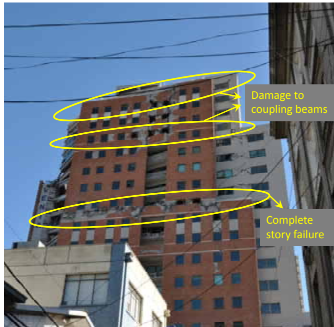
Figure 4.18 O'Higgins tower in Concepción suffered partial story collapses
