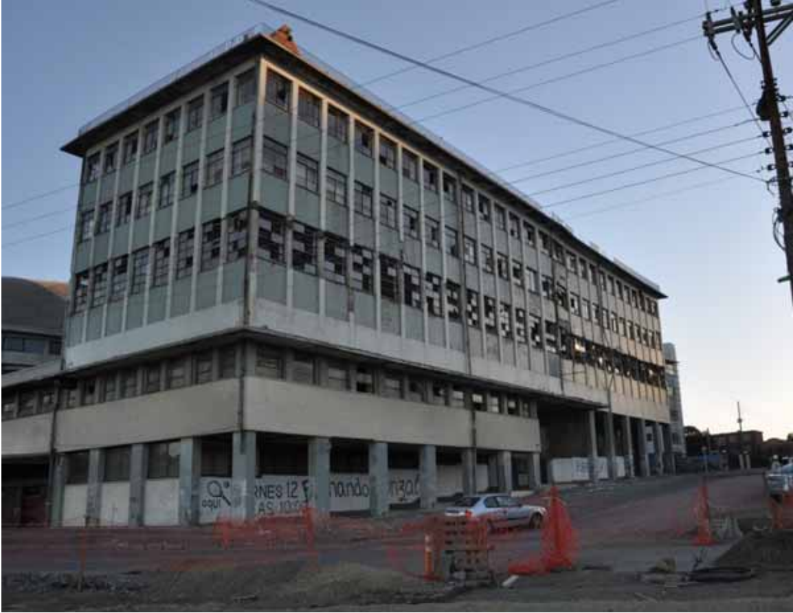
Figure 4.22 RC building near the port of Talcahuano damaged beyond repair
