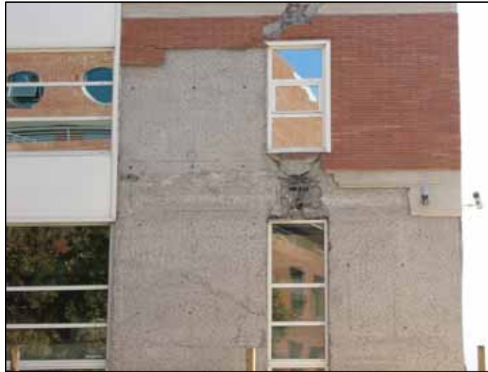
Figure 4.5 Collapsed masonry cladding wall and a damaged beam
