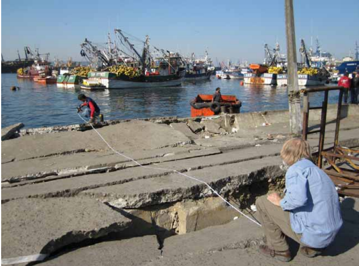
Figure 3.20 Measurement of displacement of the wall due to lateral spreading, Port St. Vicente, April 15, 2010 (-36.725517°, -73.132390°)
