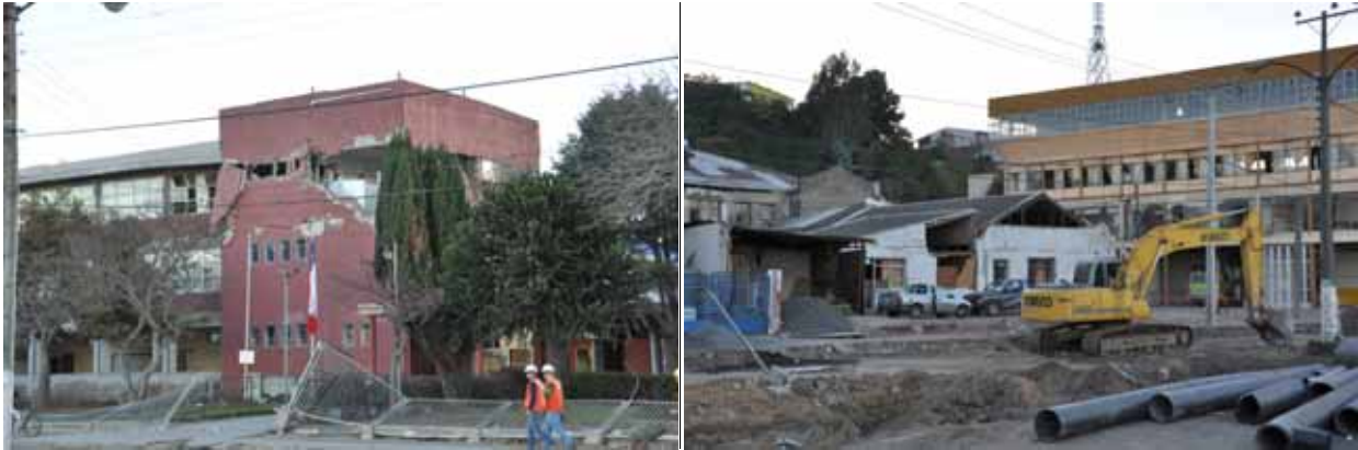
Figure 4.23 Buildings at the shorefront in Talcahuano damaged due to hydrodynamic loading
