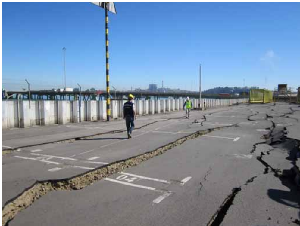
Figure 3.9 Lateral spreading looking north view 1, Port of Coronel, April 14, 2010 ( -37.028874^{\circ} , -73.149768^{\circ} )
