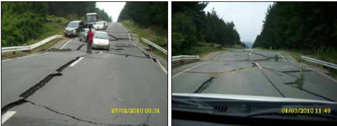
Figure 5.3 Sag vertical curve pavement failures
