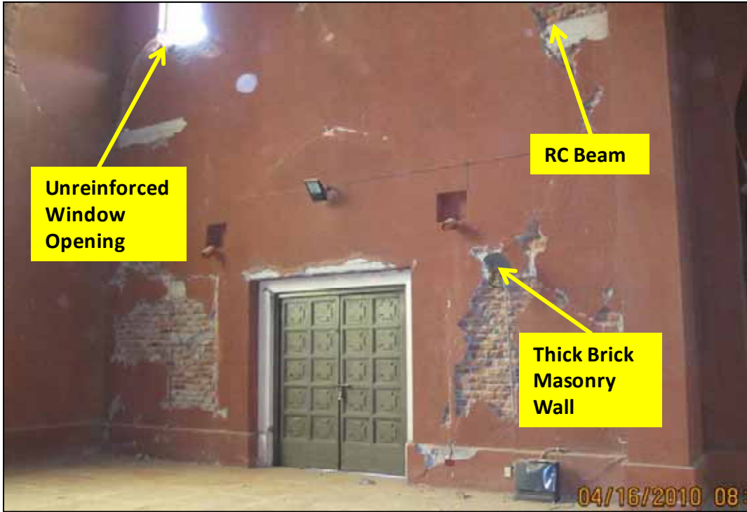
Figure 4.97 Left: Interior damage to masonry walls
