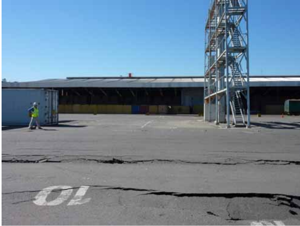
Figure 3.10 Lateral spreading looking north view 2, Port of Coronel, April 14, 2010 (-37.028874°, -73.149768°)
