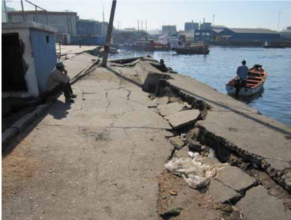
Figure 3.18 Lateral spreading and damage to quay wall, blue fish processing plants in the background damaged by lateral spreading, Port St. Vicente, April 15, 2010 (-36.725517°, -73.132390°)
