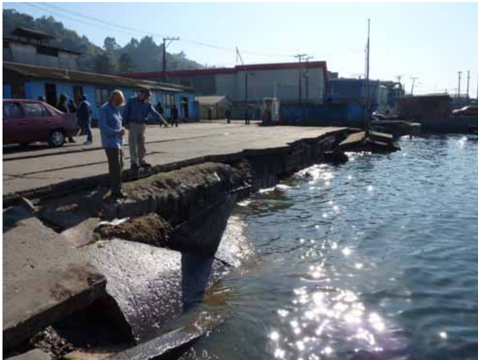
Figure 3.19 Failed section of the quay wall, Port St. Vicente, April 15, 2010 (-36.725517°, -73.132390°)
