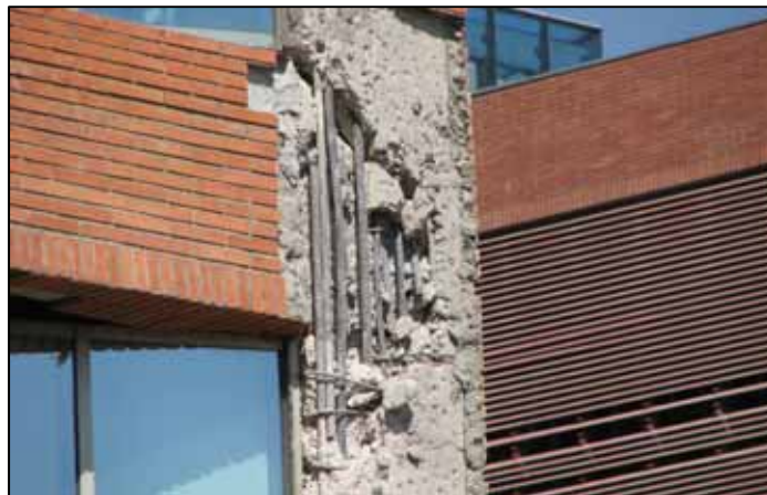
Figure 4.6 Failure of beam-column connection
