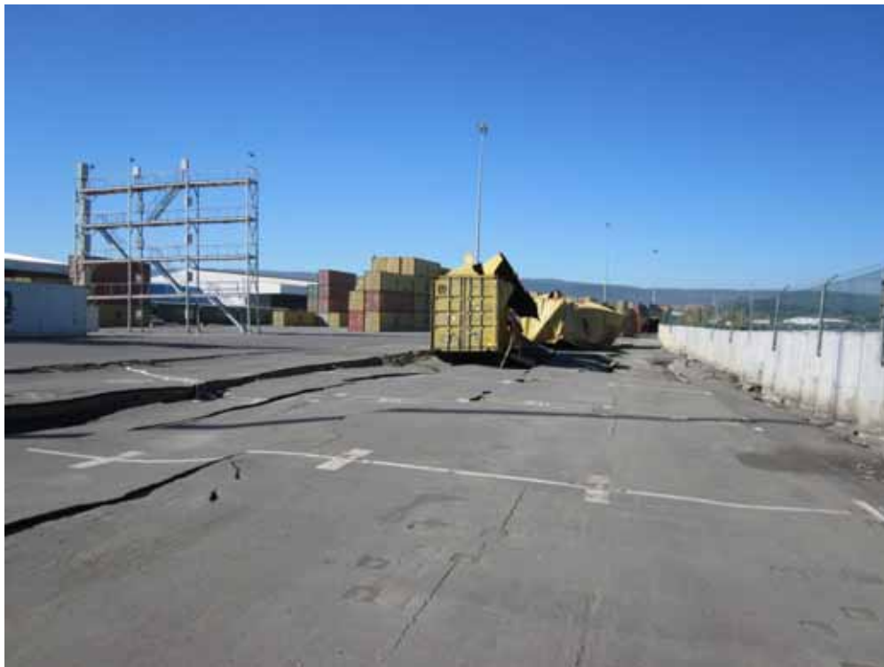
Figure 3.11 Lateral spreading looking south, Port of Coronel, April 14, 2010 (-37.028874°, -73.149768°)
