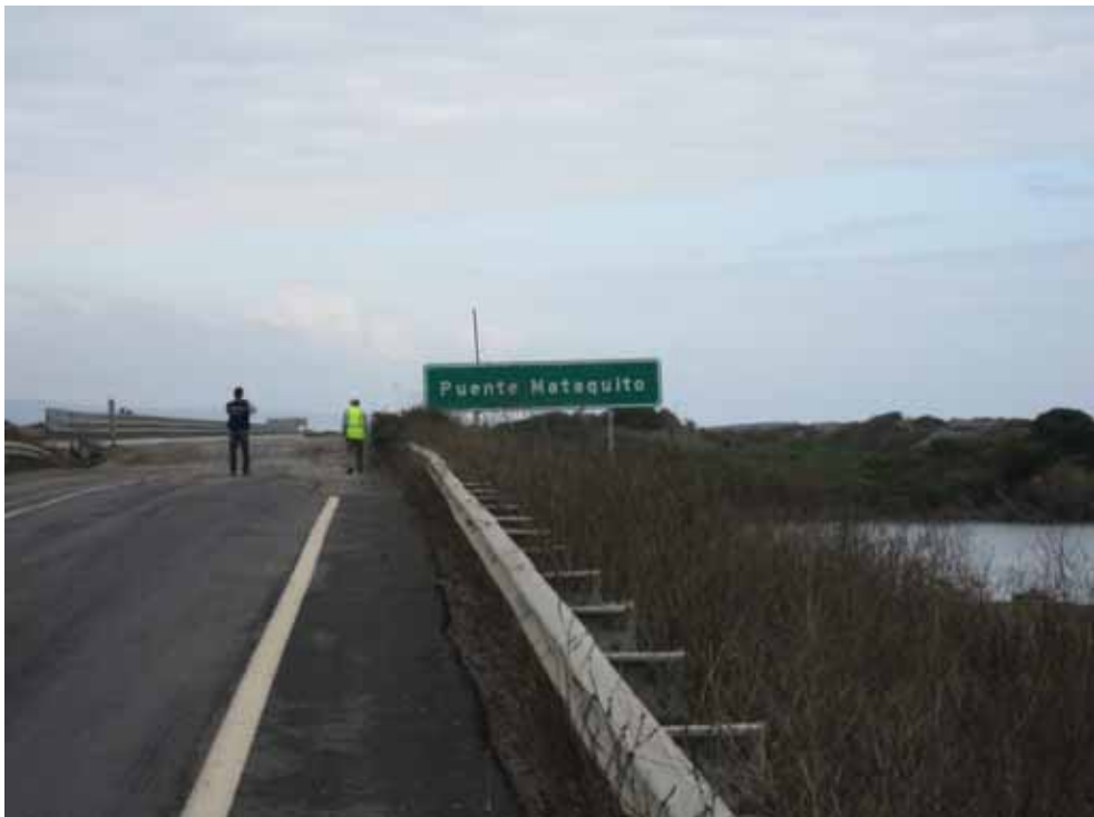
Figure 3.29 Settlement of the north abutment of the bridge, 70 cm offset at the bridge deck, Puente Mataquito, April 16, 2010 (-35.050712°,-72.162258°)
