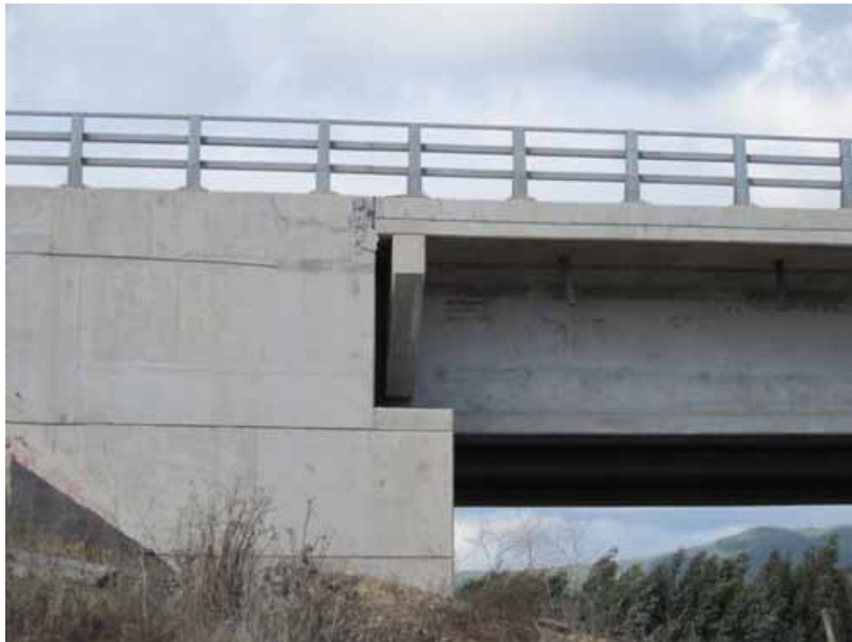
Figure 3.33 North abutment shoved into bridge deck due to lateral spreading, Puente Mataquito, April 16, 2010 (-35.050712°, -72.162258°)
