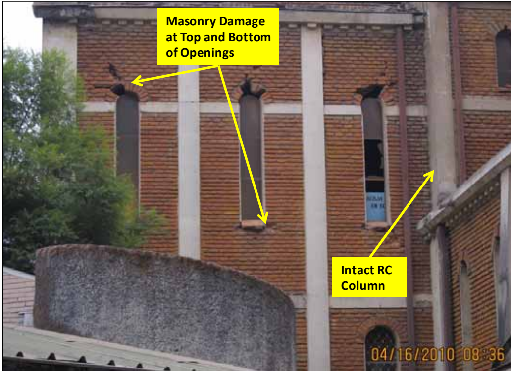
Figure 4.95 Exterior damage to masonry at corners of windows
