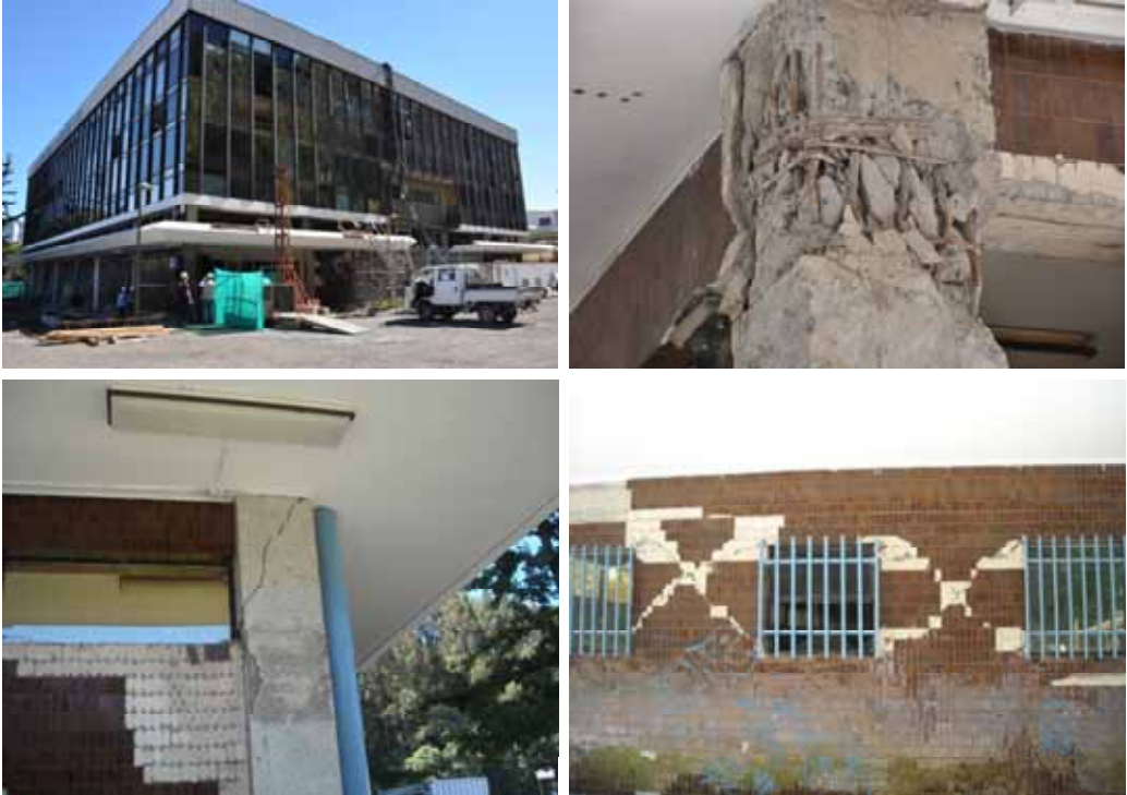
Figure 4.15 Odontology Building, University of Concepción, combined shear-compression failure at the top of first story columns, short column effect, and diagonal cracks in masonry infill walls around openings
