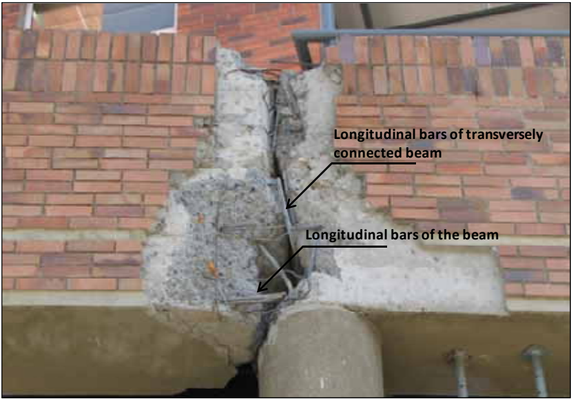
Figure 4.4 Close-up view of the damaged structure
