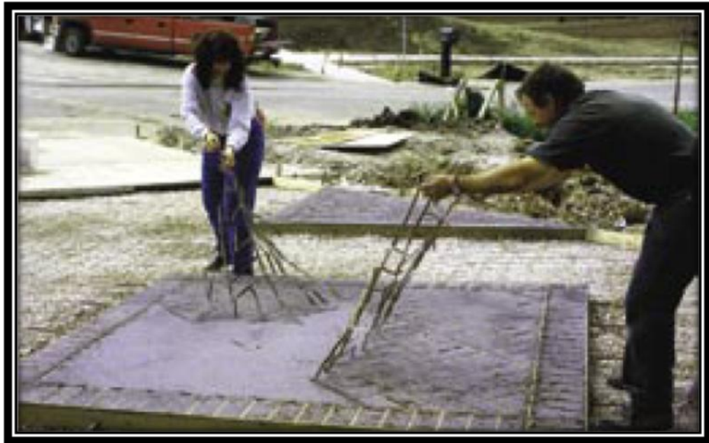
Figure 2.13 Stenciling with paper patterns on fresh concrete, applying hardeners then stencils are removed (Nasvik, 2004)
