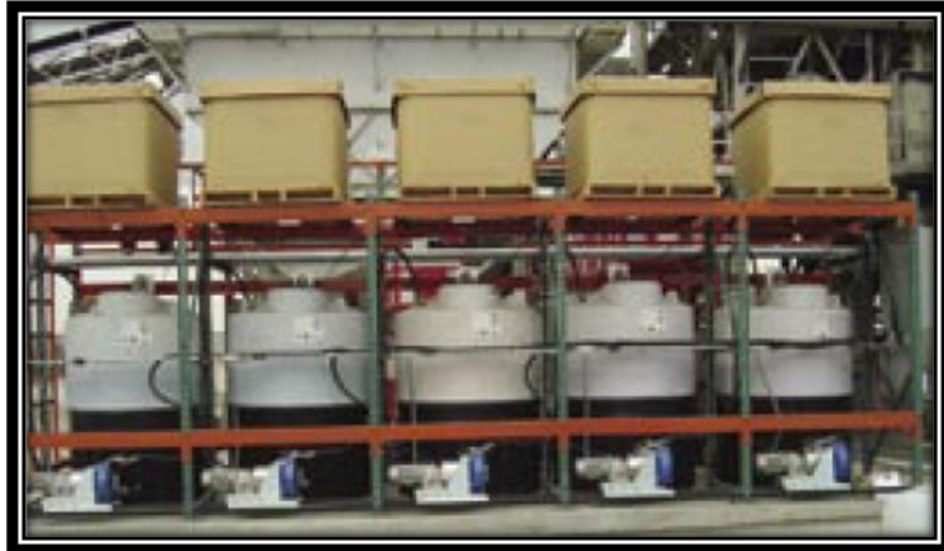
Figure 2.32 Storage tanks of primary pigments that are pumped into liquid dispensing system using a computerized program (Forgey, 2005)
