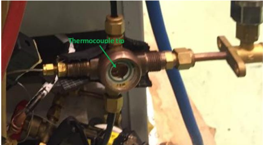
Figure 3.8: Compressor outlet thermocouple inside a sight glass.
