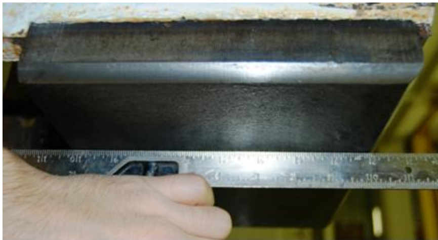
Figure 8.9 Photograph of the Bottom of a Column Base Plate After the Experimental Program Showing Lack of Damage
