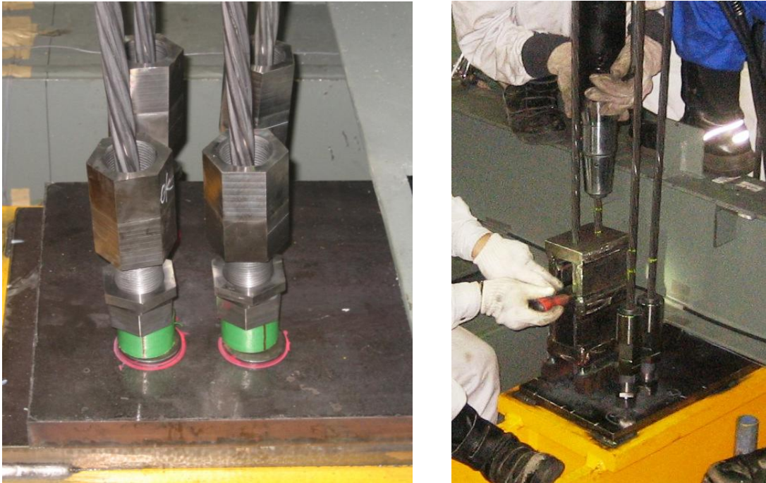
Figure 12.2 Method for Mitigating Seating Losses During Installation Including Installation of Temporary Washers (Left), and Removal of Temporary Washers (Right)
