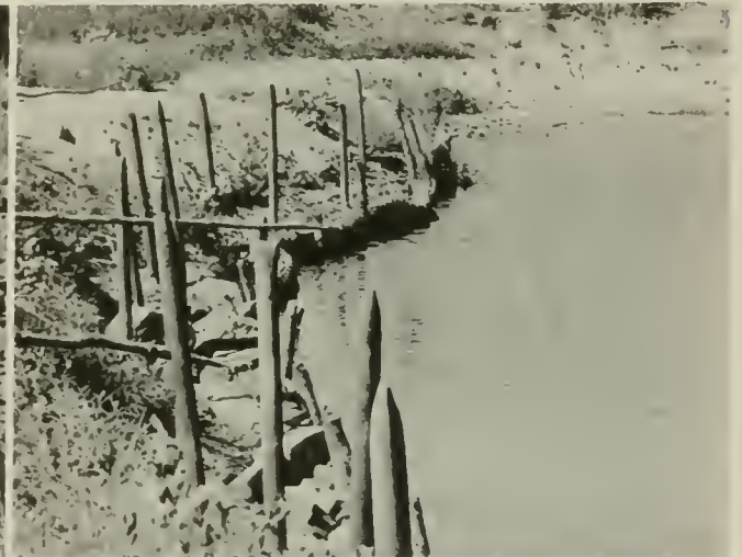
Broken concrete held in place by heavy woven-wire fencing protects the levee from crayfish and muskrats.
