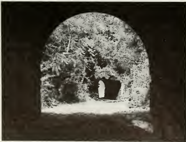
Fig. 15.—Culverts constructed of local limestone near Pearl, Pike County. These culverts supply the name—Twin Culvert Cave—for the nearby cave. An infrequently used county road and a small stream share the culverts.
