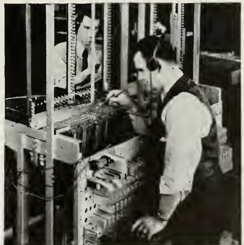
Count on a Bell Telephone switchboard too, and all the rest of the complex apparatus. Here is shown one of hundreds of inspections which Western Electric makes.
