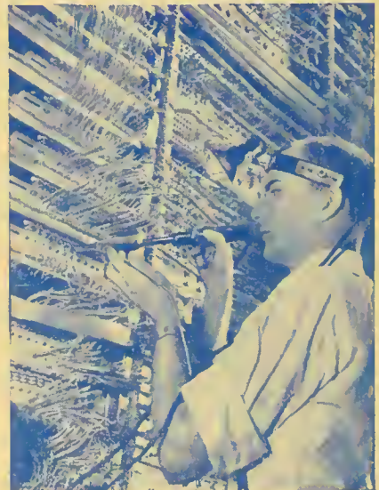
This skilled worker is performing a delicate operation on equipment for a new telephone exchange. He joins thousands of wires that will carry your voice wherever there are telephones.
