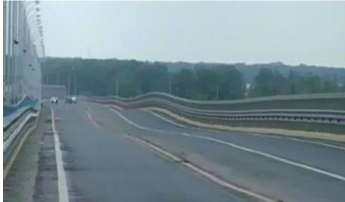
Figure 1.1.1 Vortex-induced vibration in the Volgograd Bridge 1)
