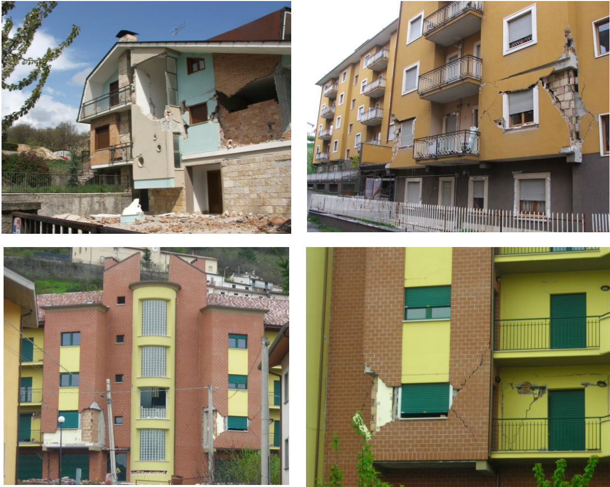
Figure 1 – Collapse of non-structural components in residential reinforced concrete (RC) multi-storey framed buildings in the outskirts of L’Aquila during the 6 April 2009 (Italy) earthquake, designed according to allowable-stress ( top ), limit state ( bottom ) seismic codes .
