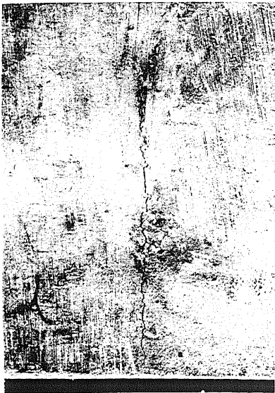
(c) CRACK NEAR WELD. 1.5X
