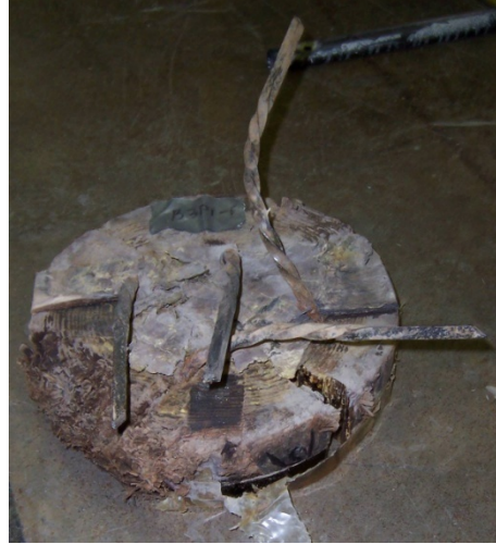
Figure 4. Damaged "post" connection.
