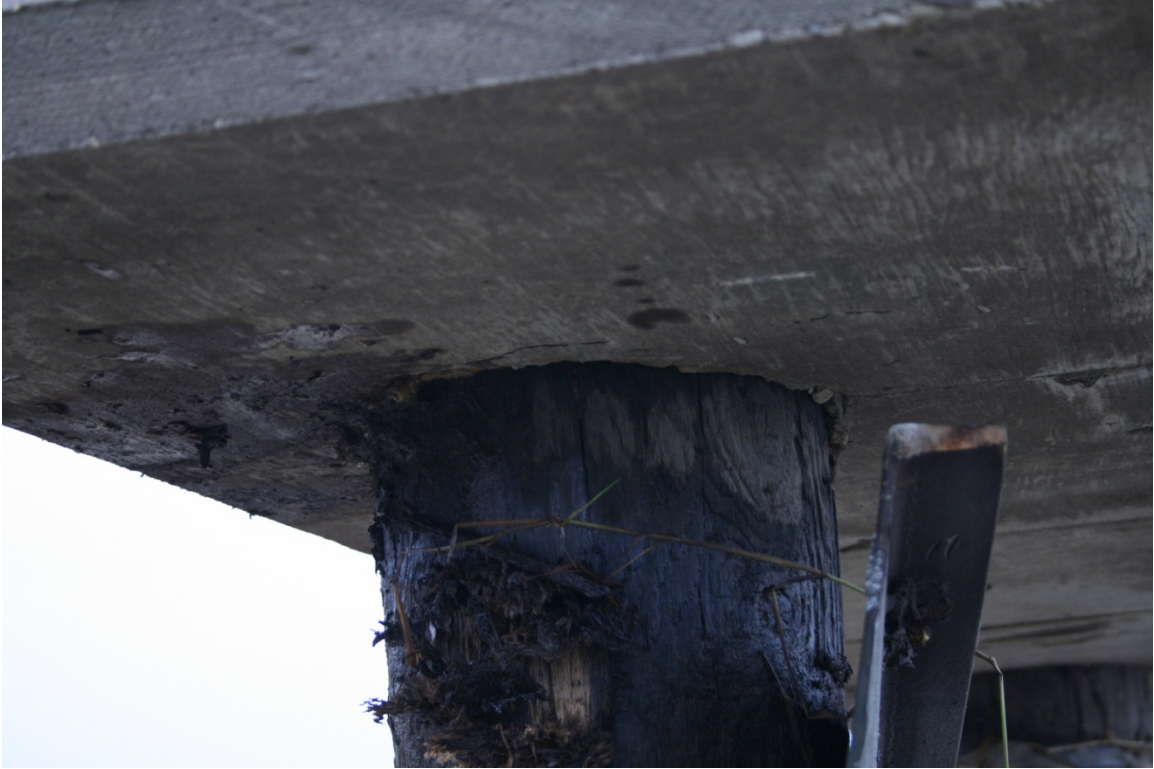
Figure A-10. Intact pile to pile cap connection after collapse.
