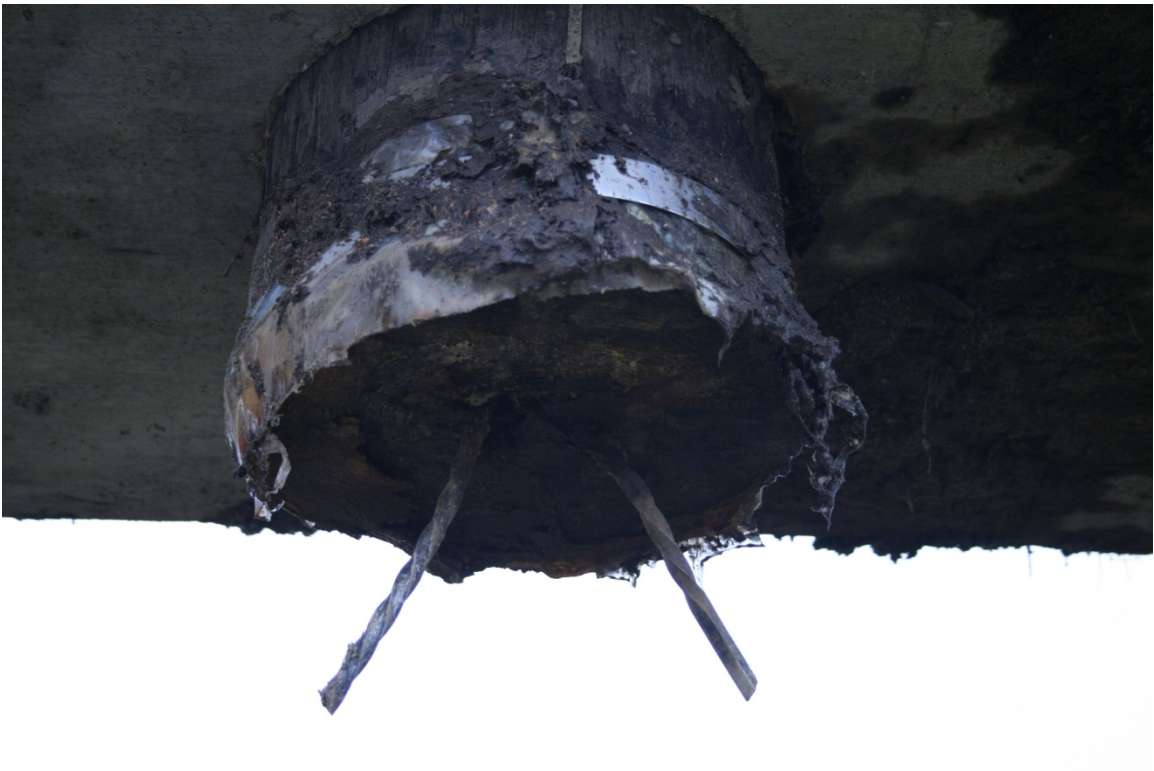
Figure A-11. Failed post connection.
