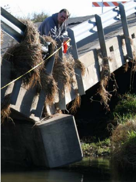
Figure A-5. Collapsed bent 3 pile cap.
