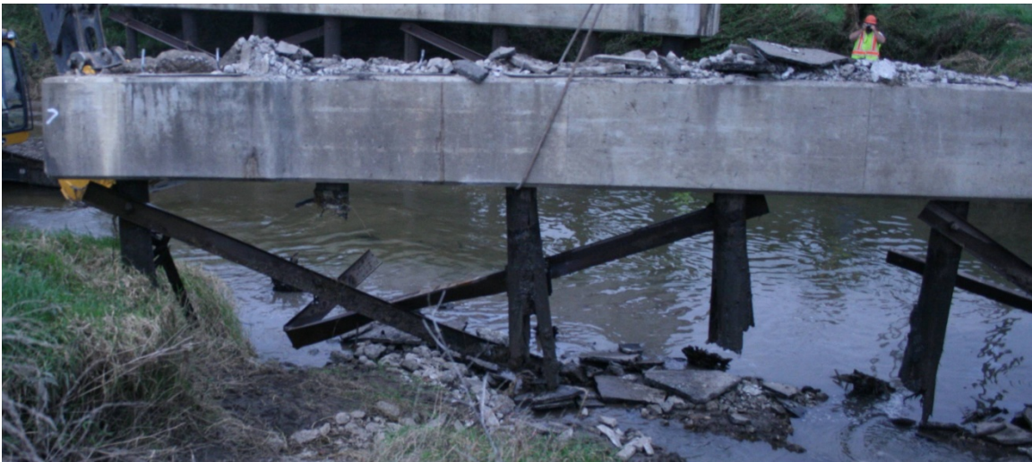
Figure A-8. Fractured piles and failed post connection.
