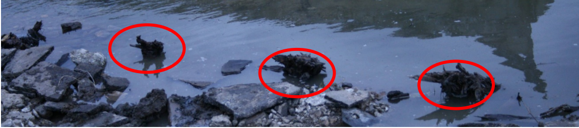
Figure A-12. Piles remaining in riverbed.
