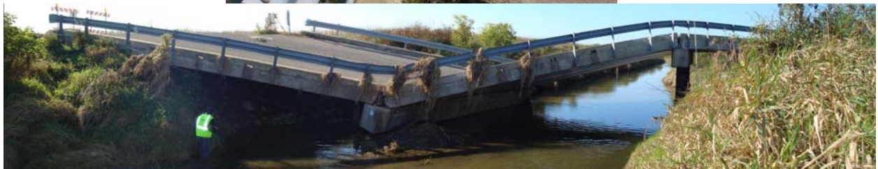
Figure 5. Illinois Dekalb County Bridge No. SN019-5010 after collapse.
