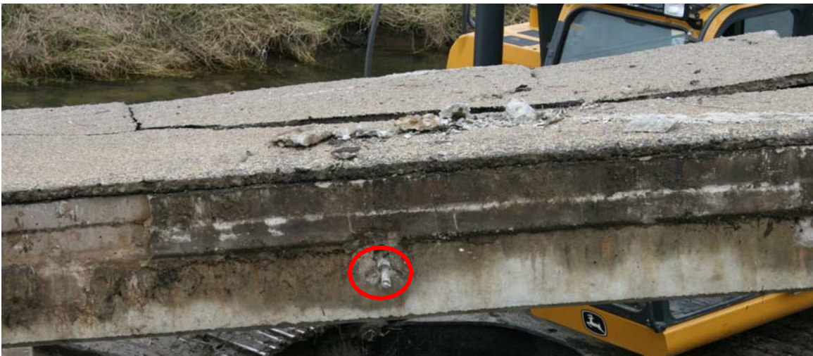
Figure A-1. Deck beam with transverse ties cut.
