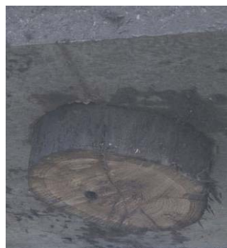
Figure 6. Typical pile-to-pile cap connection in bent 3 after collapse.
