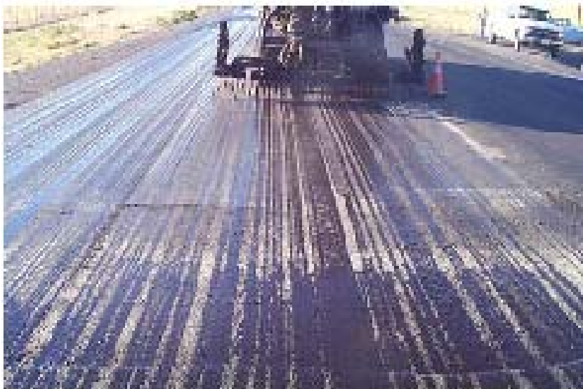
Figure 3-7. Uneven zebra tack coat distribution.
