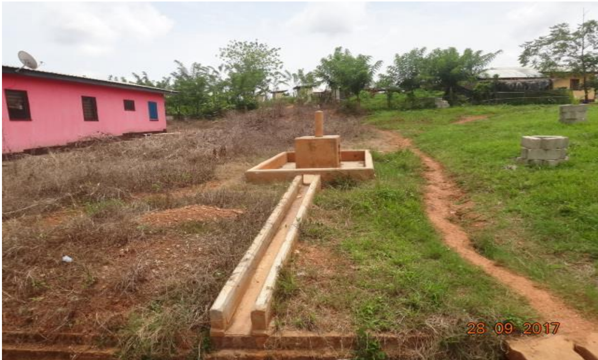
Figure 7.7 An abandoned and rusting water system in Community C
