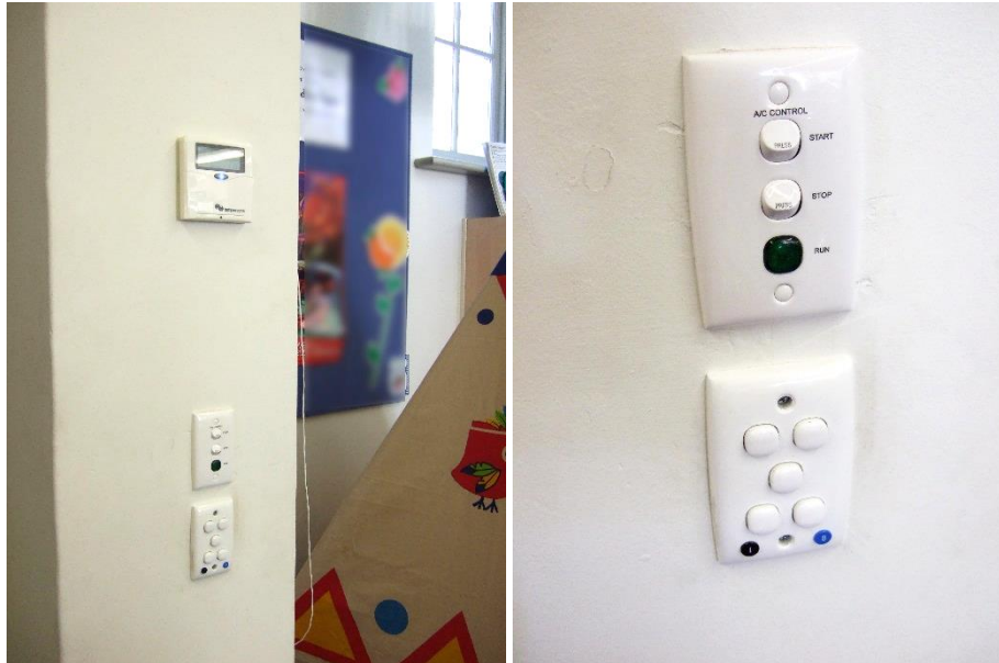
Photograph 4.8: Typical local controls, Red.3 shown – left, HVAC set point control above, with controls below (DSCF6477_120802mod.JPG); right, detail of controls, HVAC f above, lights below (DSCF6476_120802mod.JPG).
