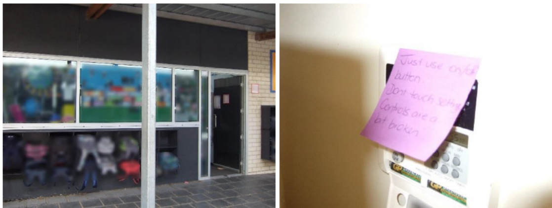
Photograph 6.1: Ventilation and HVAC controls with local adaptations: White.3 door propped open in winter (DSCF6281_120730mod.JPG), and Yellow.2 HVAC instructions (DSCF6058_120326mod.JPG)
