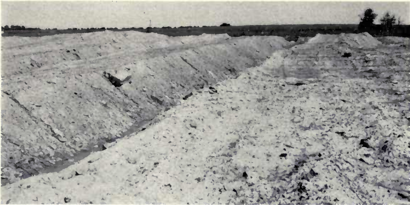
All ridges have been topped to a width of 12 to 16 feet with a bulldozer. The area is now easily accessible. (Fig. 25)
