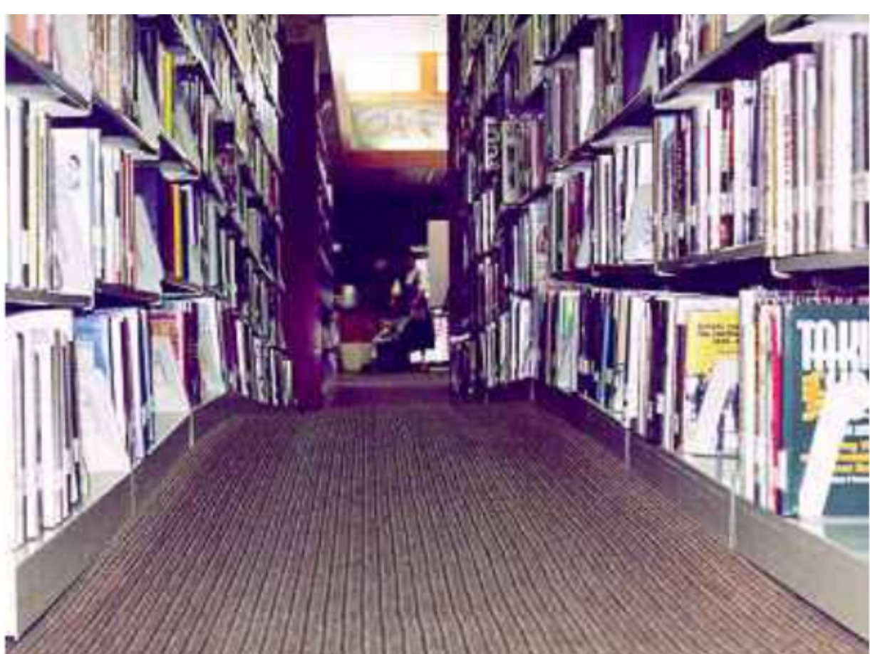
Fig. 6 - Example of heaved floor at Johnson City Public Library (USA) [3].
