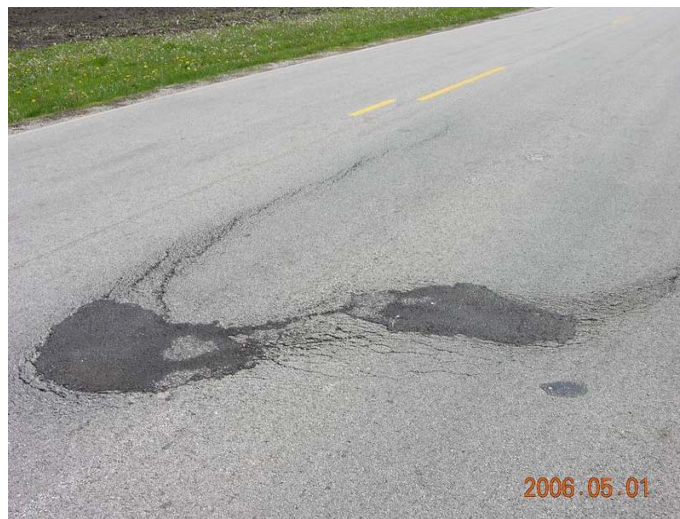
Figure 1-1. Slippage cracking caused by poor interface bonding.
