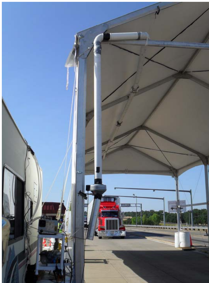
Figure 2. Photograph showing a closer view of the exhaust sampling pipe anchored to the roof of the tent. The inline fan is the metal oval between the two sections of pipe.
