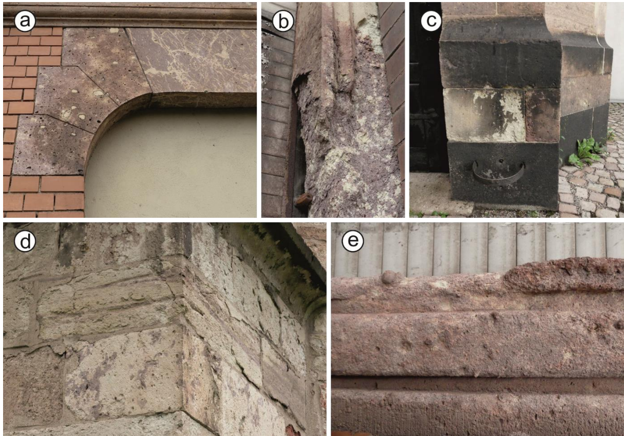
Figure 6.2: Appearance of different damage and deterioration types observed in the Hilbersdorf Tuff. a Loss of components displays the most observed type of deterioration at the Precious Tuff (HP). b Back-weathering due to crumbling and scaling of the Regular Tuff (HR) variety in a door jamb. c Discoloration in the splash zone of water at the castle church of Chemnitz. d Scaling of the Sculpture Tuff (HS) and Regular Tuff (HR) variety at the collegiate church in Chemnitz/Ebersdorf. e Loss of matrix that results in protruding lapilli components in the Lapilli Tuff (HL) observed in a door jamb
