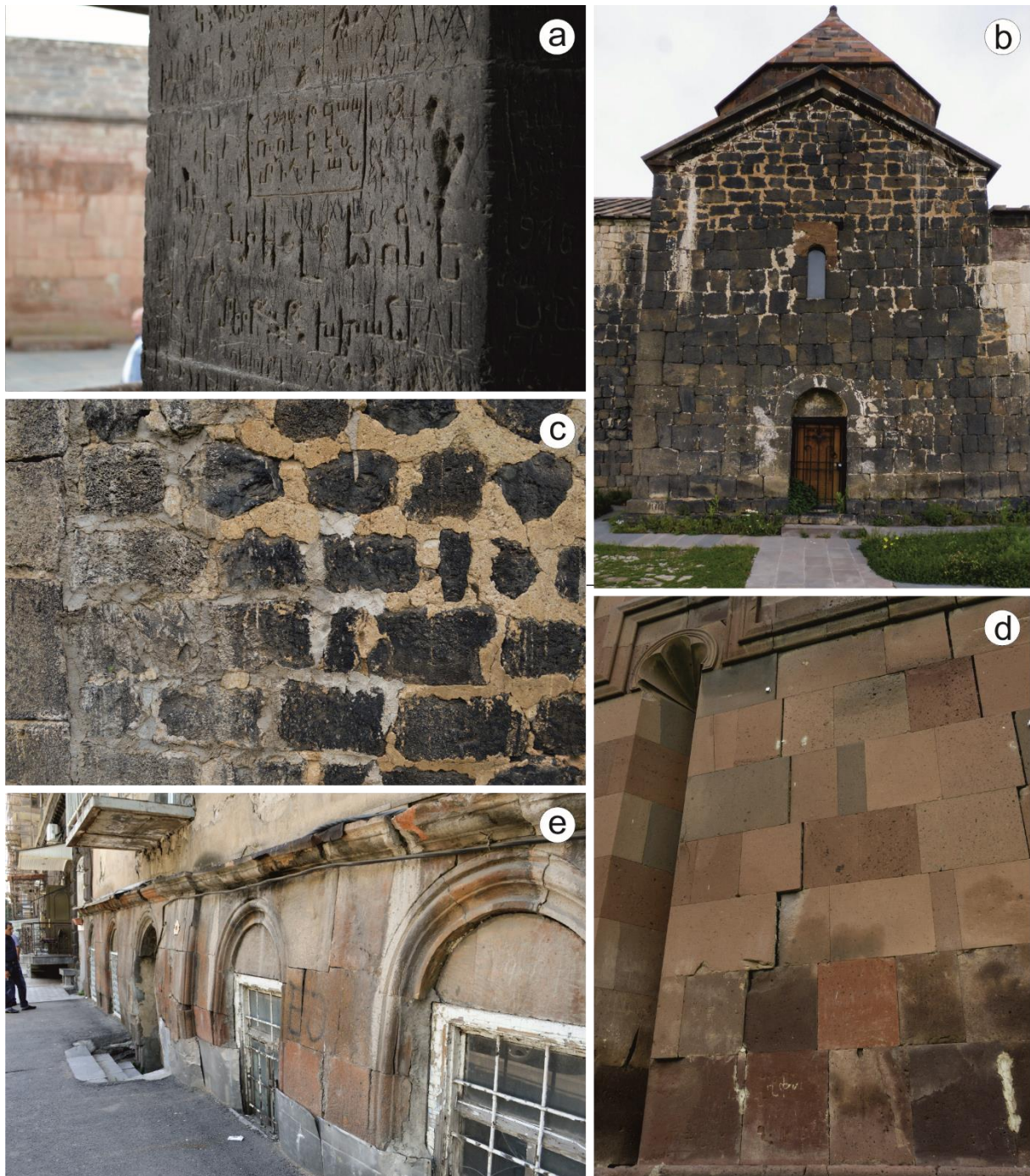
Figure 4.6: Different forms of deterioration due to anthropogenic and natural hazard causes: a Man-made carvings at the facade of the Khor Virap monastery. b, c Inadequately executed mortar repairs at the Sevanavank monastery. d, e Earthquake-related crack formation and deformation of tuff facades
