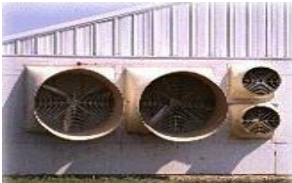
Mechanical ventilation in grow-finish building (Source: Purdue University)
