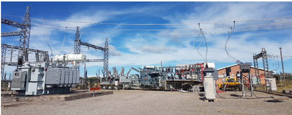
Figure 2.6: 132-66 kV/22-11 kV Mobile Substation
