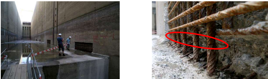
Figure 8: Lock chamber wall with the exposed section directly above the bottom of the lock (left); fractured rebars in the construction joint (right)
