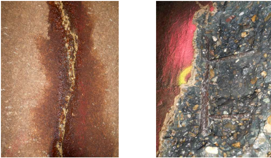
Figure 12: Calcium carbonate deposits at the leaking vertical crack (left); rebars exposed near the vertical crack (right)
