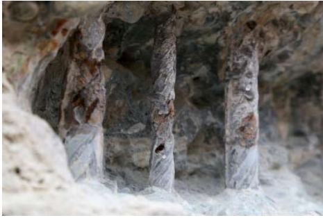
Figure 10: Corroded rebars in the construction joint
