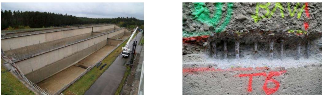
Figure 9: View of the side ponds of the lock (left); exposed rebars in the leaking horizontal construction joint of the wall between the two side ponds (right)
