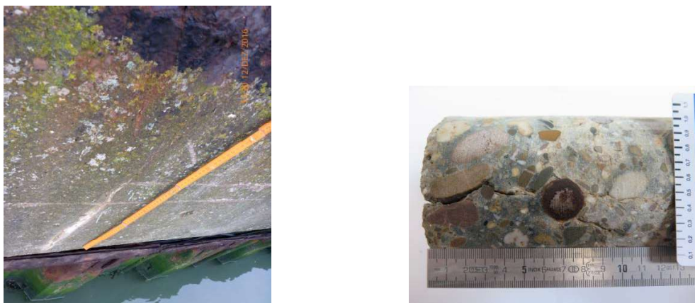
Figure 3: Continuous crack on the face of the quay with calcium carbonate deposits near to where drilled core no. 4 was taken on the top surface (left); drilled core no. 4, 1st layer of rebars, concrete cover approx. 60 mm (right)
