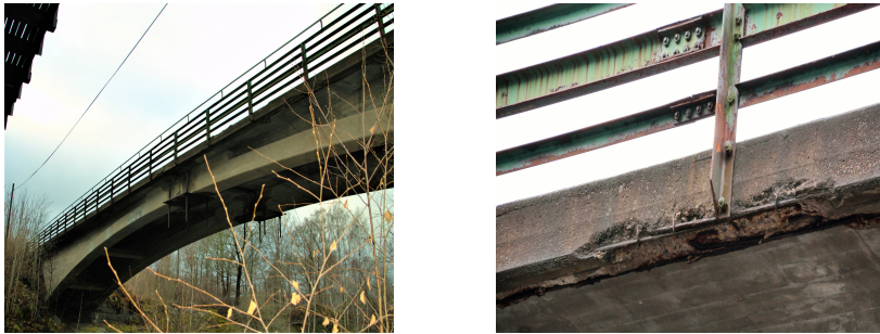
Figure 3.1: Gullspång bridge: view of the bridge before demolition (left) and exposed tensile reinforcement bars and spalling in an edge beam (right). Photos courtesy of Ignasi Fernandez
