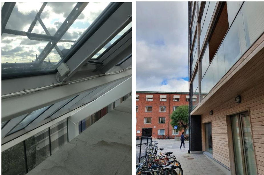
Figure 4.20. There were some problems with rain leakage around windows (left), glazed balconies (right).
