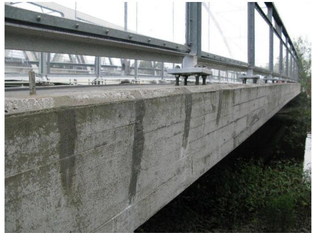
Figure 1. A bridge edge beam in Sweden with cracks that have been injected and sealed.
