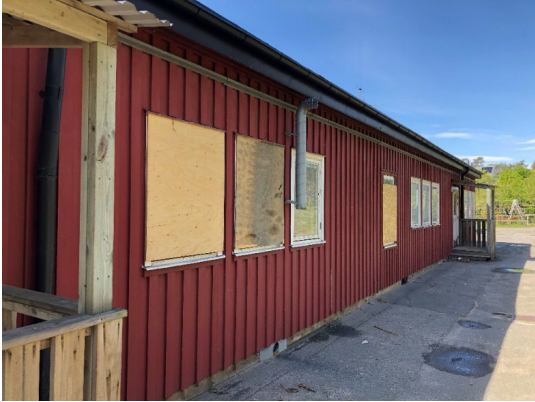
Fig. 1 A typical school building with a crawl space and indoor air quality problems
