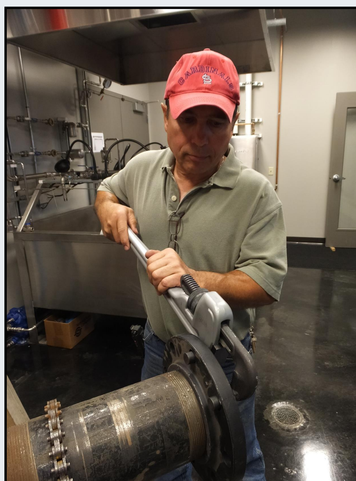
Figure 1: Pipefitter using a pipe wrench to undo nuts on a pipe flange
