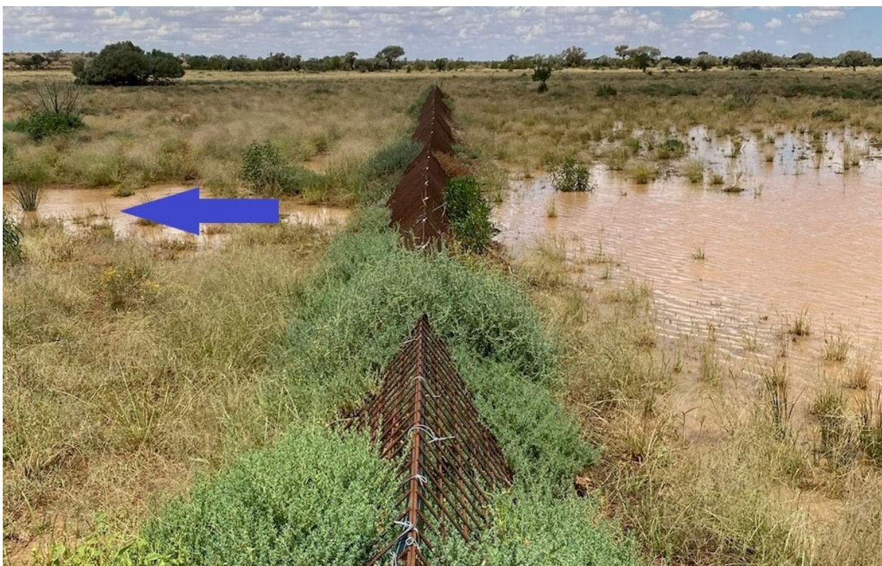
Photo 2: A variety of techniques are used in the identified priority projects. This sieve structure on Allandy protects the exit point of an ephemeral wetland. The innovative triangle-shaped design makes it robust and provides a protected niche for plant establishment. Blue arrow indicates flow direction.
