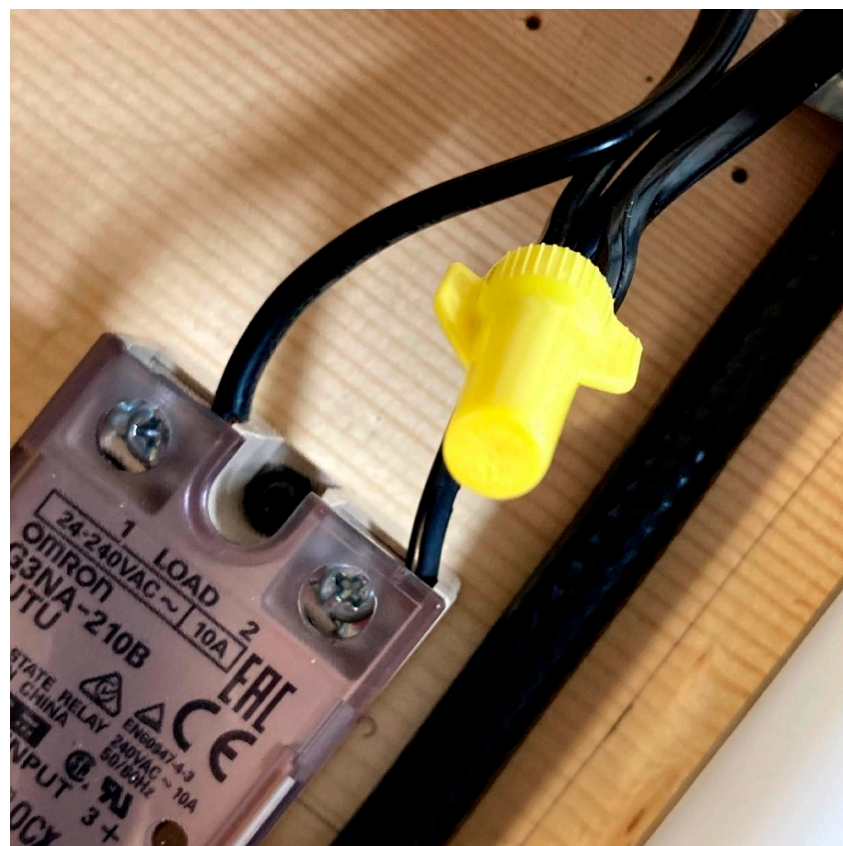
Figure 13. The power cable was secured into the load terminals of the relay.
