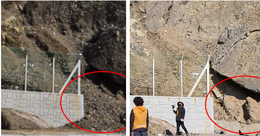
Figure 13. Sediment erosion between the concrete wall and boulder
