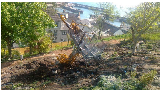
Figure 3 Soil nailing rig positioned on site. A short section of soil nail can be seen on the slope in front of the rig.
