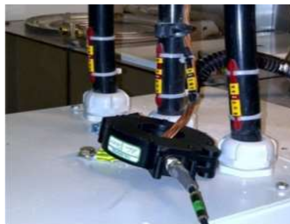
Fig. 6. Measurement of PD signal with HFCT at HVPD Ltd.
