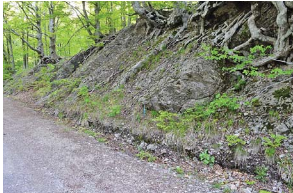
Figure 10: The Main Dolomite strata with a thickness of 30 – 110 cm in the cutting of Majstorska Cesta, on the N slope of the Mali Alan Pass (scale – geological hammer is 31 cm long)
