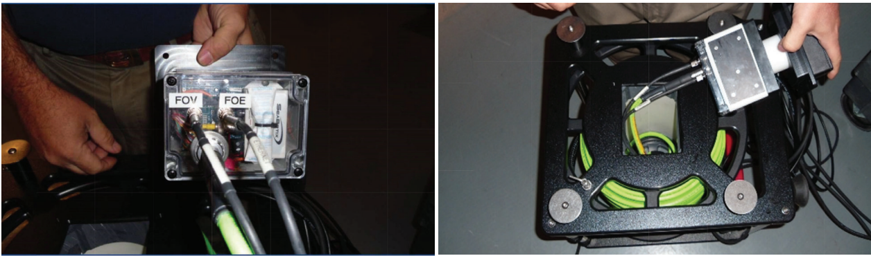
Figure 10 The Cable line drum with the optical signals to electrical signals converter Slika 10. Bubanj s kabelima s pretvaračem optičkih signala u električne signale
