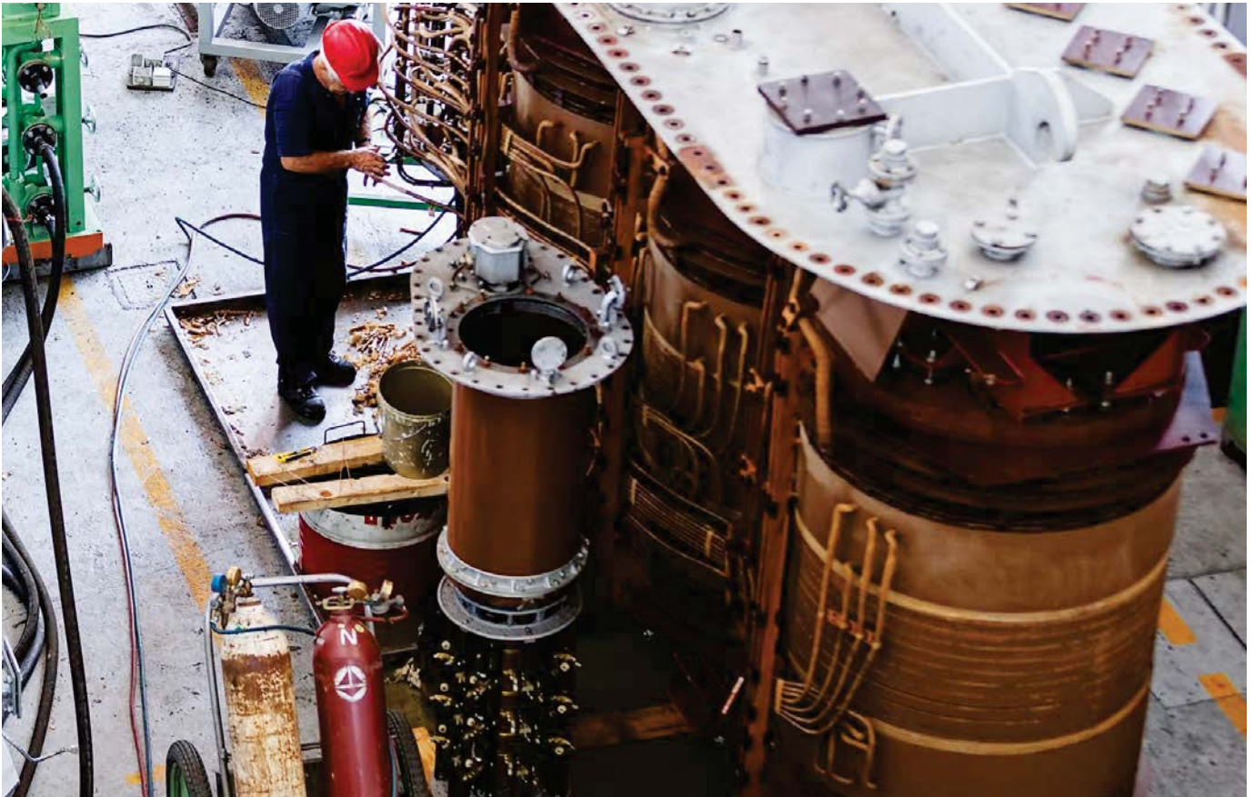
Active part inspection
