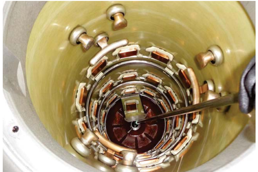
Internal inspection of an OLTC
