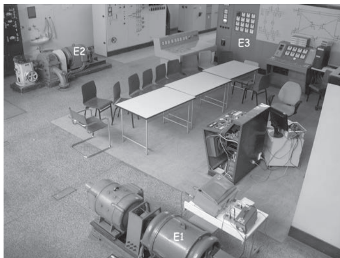
Figure 1. Part of power system laboratory
