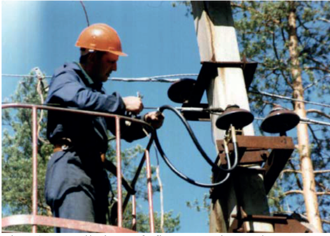
Fig. 4. Installation of first experimental arresters (LFA-Ls) in St. Petersburg utility (Russia) in 1999.
