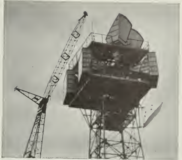
Microwave relay towers assure reliable land transmission of telephone, radio, television and data traffic—with complete flexibility.
