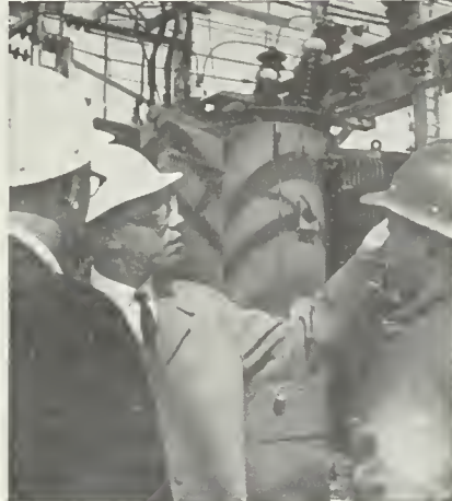
JACK LAMBERT, E.E., KENTUCKY '60 —Jack works on design, installation, and maintenance of power stations, distribution networks, motors, and drive systems at our Steelton, Pa., Plant.
