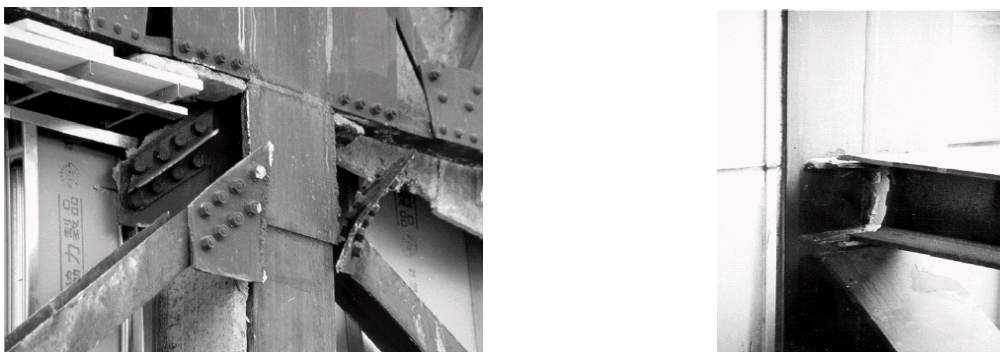
Figure 2.12. Damage to nonductile braces in the Kobe earthquake: fracture of welded connections and web tear-out ( left ) and fracture of welded connections ( right ) ( after Naeim, 2001).
