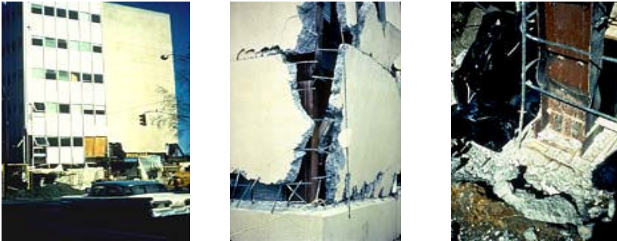
Figure 2.2. Cordova building damaged during the 1964 Alaska earthquake: overall view ( left ), local buckling in columns with ( middle ) and without RC wall ( right ) ( after NISEE, 2000 ).
