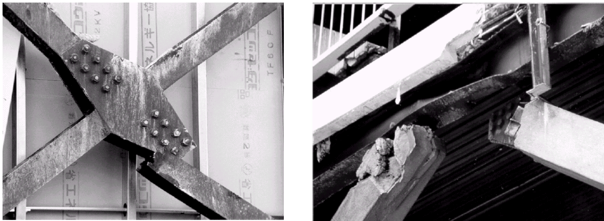
Figure 2.11. Damage to nonductile braces in Kobe earthquake: net fracture at bolt holes ( left ) and severe distortion of unstiffened beam in chevron braces ( right ) ( after Naeim, 2001).
