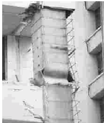
Figure 2.4. Local buckling in box column of Pino Suarez high rise buildings in Mexico City (after FEMA 355E, 2000).
