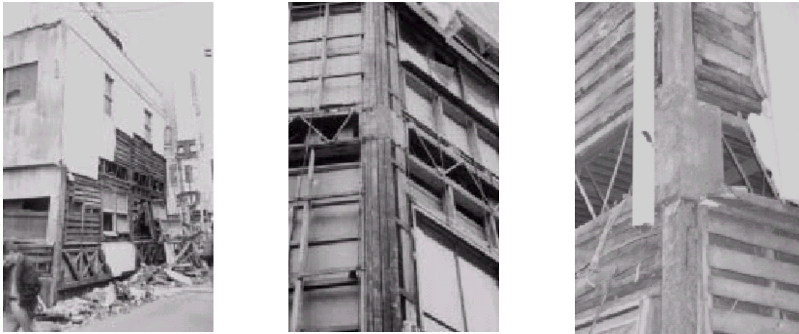
Figure 2.8. Damage to old steel buildings in the Kobe earthquake: collapse ( left ), construction with light gauged sections ( middle ) and corroded sections ( right ) (after FEMA 355E, 2000).
