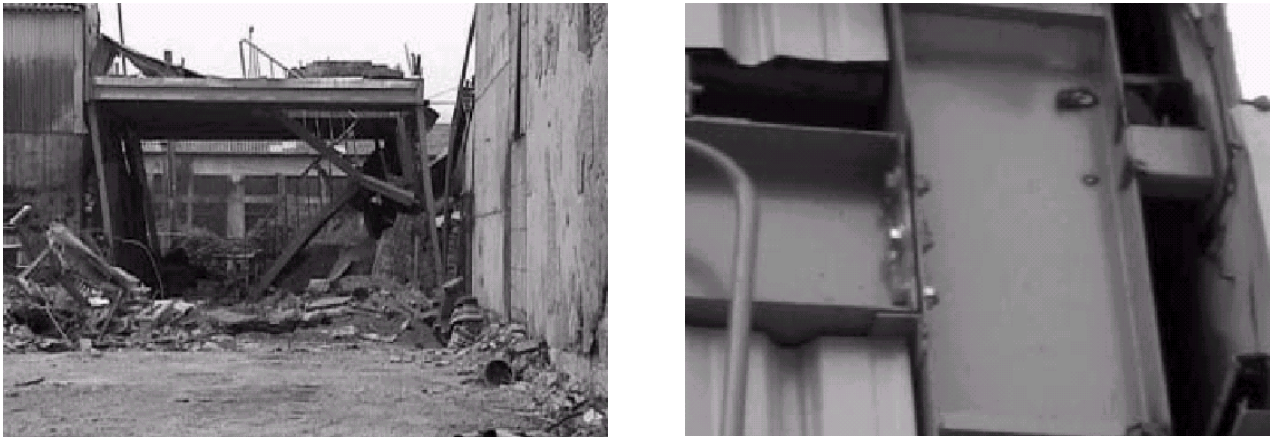
Figure 2.15. Damage in Taiwan earthquake: permanent lateral displacement in small steel frame ( left ) and yielding in the connection of light steel frame ( right ) (after FEMA 355E, 2000).
