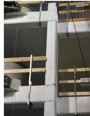
(c) Cracks on Col 6
