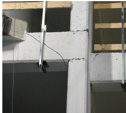
(b) Crack on beam 5
