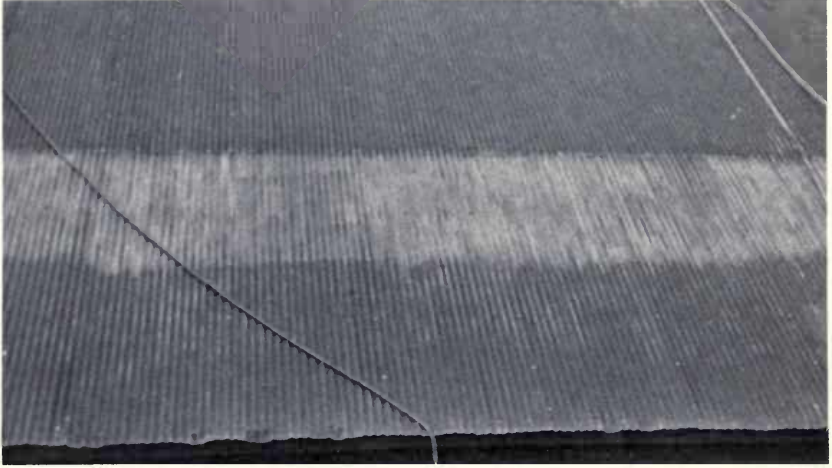
The top portions of the bottom sheets of Panels 46 through 81 on the north side were wire brushed before painting. These panels were 100 percent rusty (see Fig. 2). (Fig. 10)
