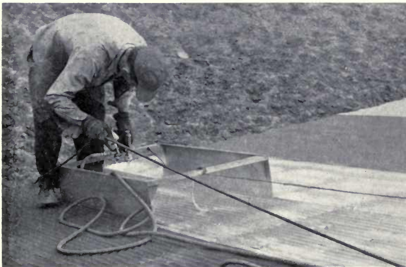
An aluminum shield was used to prevent spray from blowing to adjacent panels. (Fig. 3)
