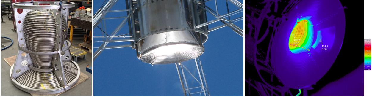
FIGURE 2. The SG4 receiver, before insulation, and then installed and in operation. Peak temperatures observed are at the pipe restraints within the cavity.
